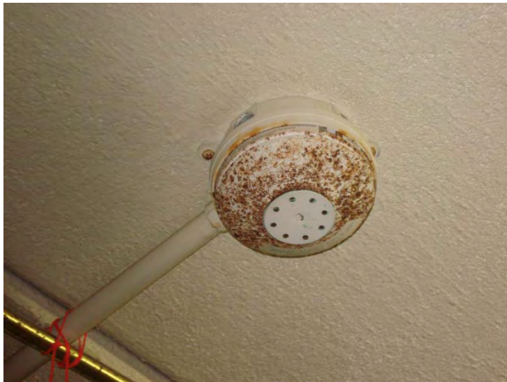
Photo 7: Filter Building Smoke Detector Corrosion
