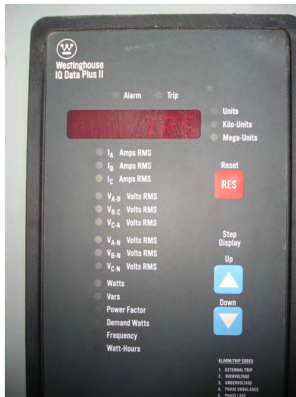
Photo 2: Switchboard Power Monitor
