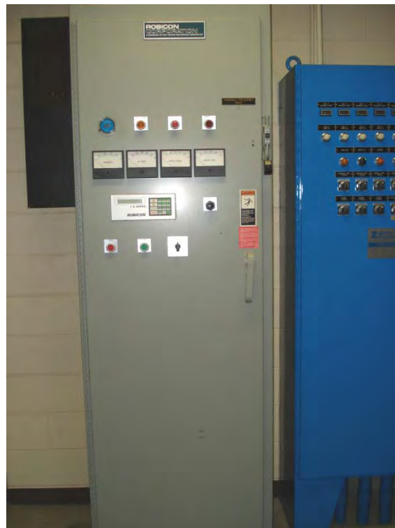
Photo 4: Robicon VFD for Effluent Pumps
