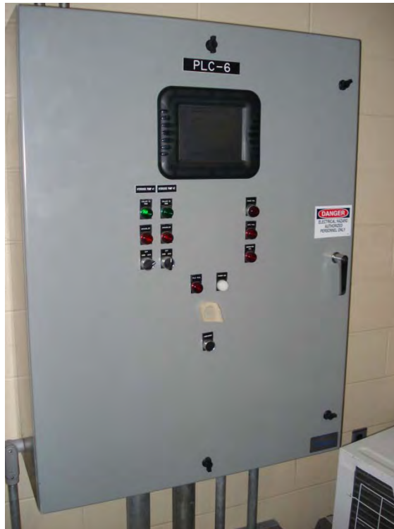
Photo 4: Filter Building SCADA System Panel
