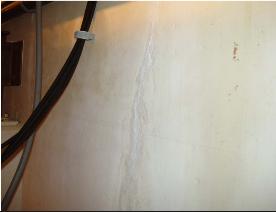
Photo 7: Clearwell Gallery Wall Surface with Efflorescence.
