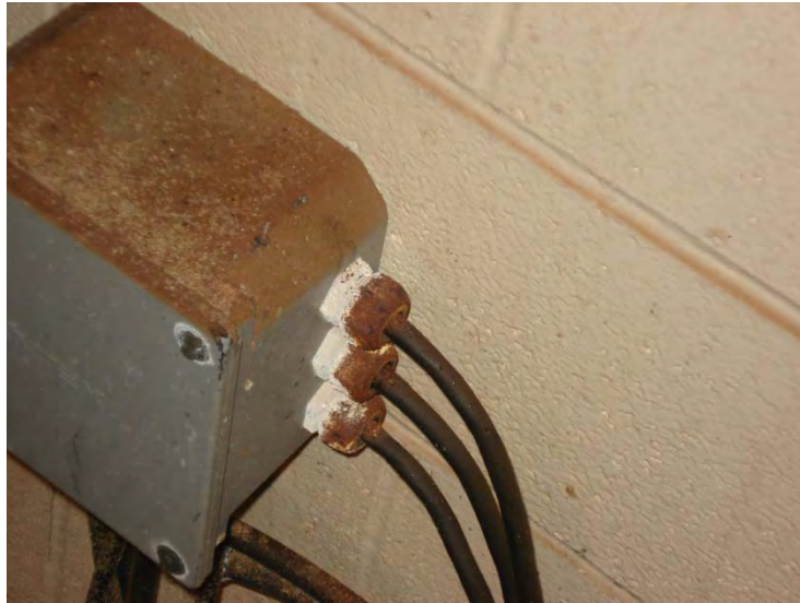
Photo 6: Filter Building Raceway Corrosion
