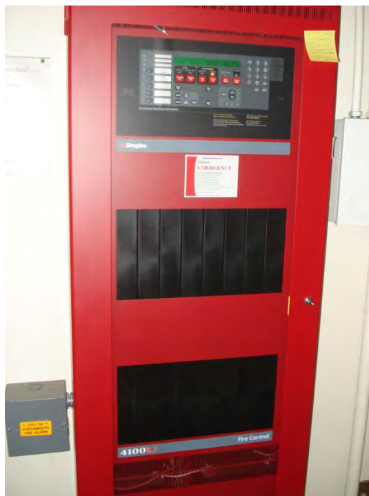
Photo 5: Control Building Main Fire Alarm Panel
