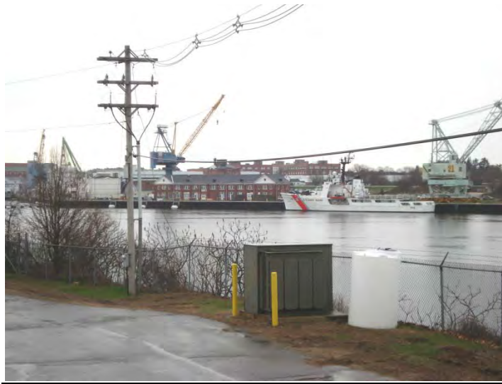
Photo 1: Utility Riser Pole and Transformer
