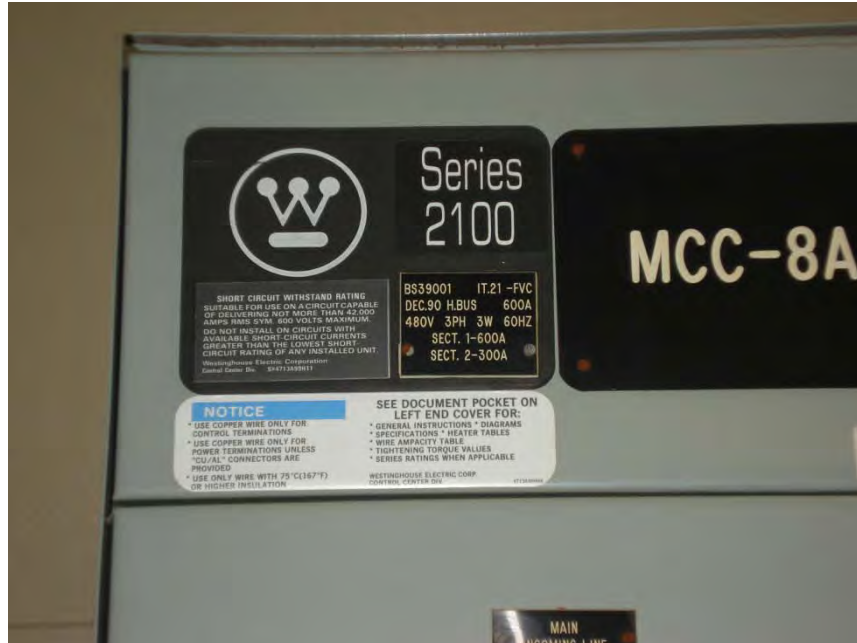
Photo 3: Motor Control Center Data Nameplate
