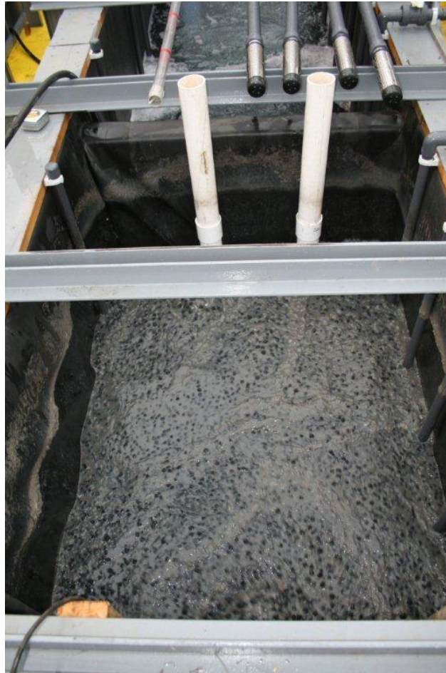
Figure 2-7 MBBR Aeration Tank
