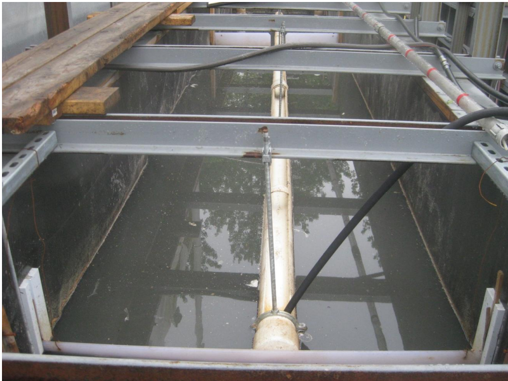
Figure 2-3. Pilot Primary Clarifier
