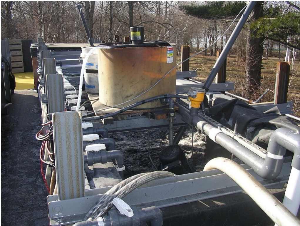
Figure 2-5. CAS with BioMag Aeration Tank
