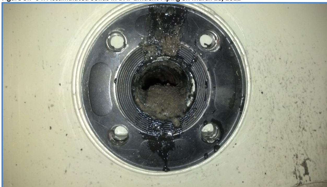
Figure 3.7-04: Accumulated Solids in DAF Effluent Piping on March 28, 2012
