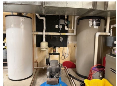
Upgraded hot water heater. Image: Courtesy of CRH.
