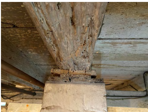
9 – Decayed timber on masonry pier
