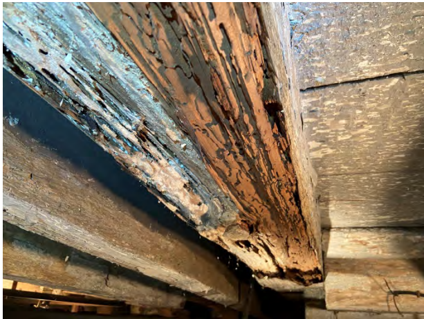
7 – Decayed timber joist
