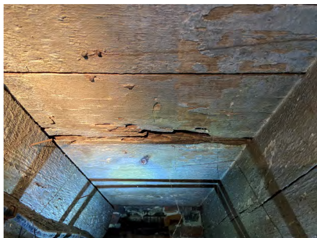
10 – Area of decayed floor deck
