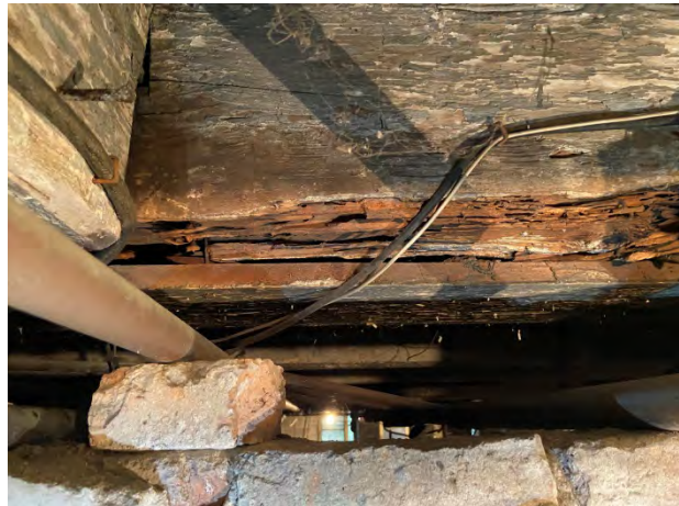
8 – Decayed timber joist
