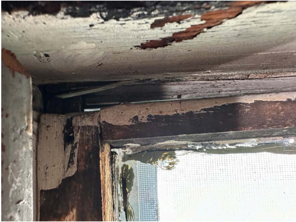
Image #39. WORN WINDOW FRAME OPEN TO OUTSIDE ELEMENTS ATTIC FACING HOLMES COURT
