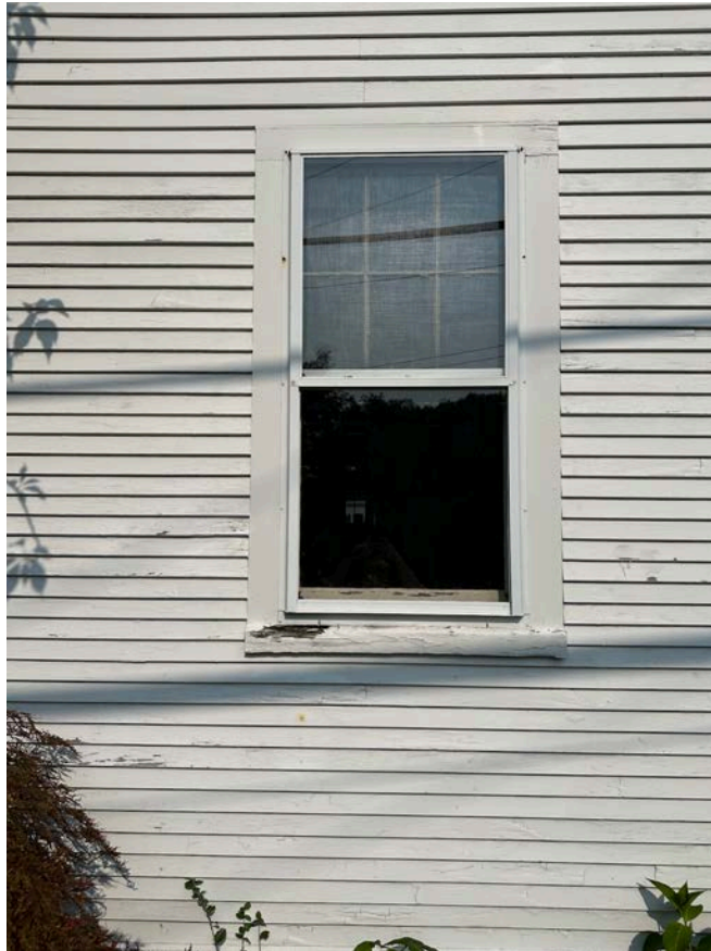
Image #33. ROTTEN FIRST FLOOR WINDOW SILL, DAMAGED STORM WINDOW, AND TRIM WORK FRONT ELEVATION
