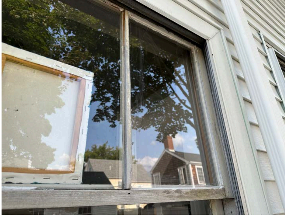
Image #41. LOOSE GLAZING AND WINDOW MUNTINS REAR ELEVATION
