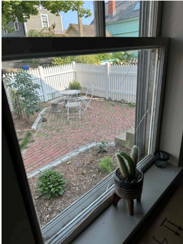
Image #43. CRACKED WINDOW PANE REAR ELEVATION, CENTER
