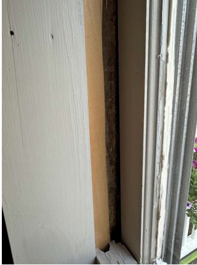
Image #47. MISSING ROPE AND WEIGHT MECHANISM REAR ELEVATION
