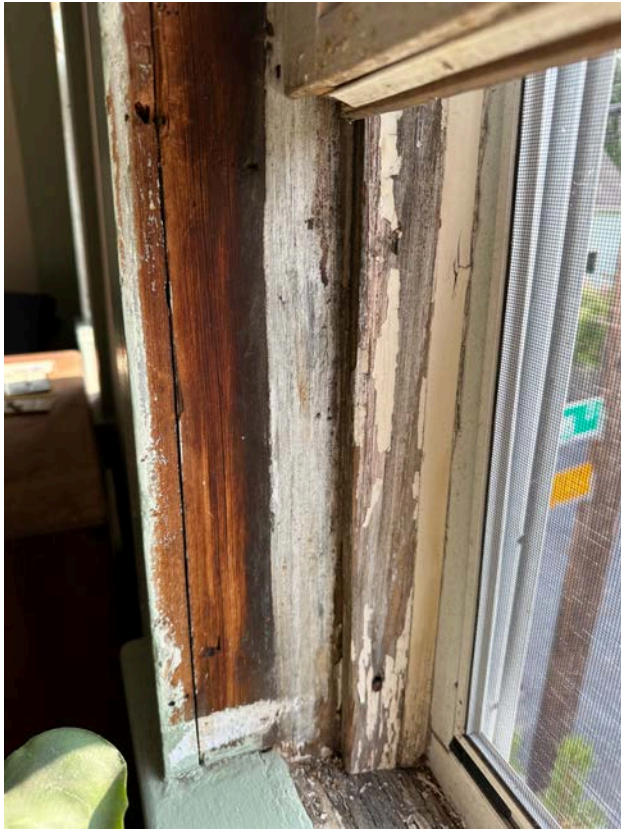
Image #59. MISSING TRIM WORK ON WINDOW FRAME, FROM INTERIOR FRONT ELEVATION
