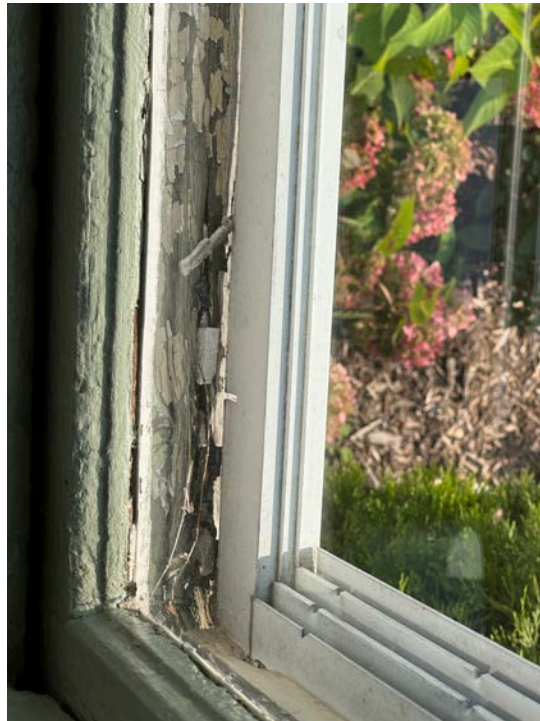
Image #54. ROTTEN WINDOW FRAME AND SEPARATION FROM STORM WINDOW, FROM INTERIOR FRONT ELEVATION
