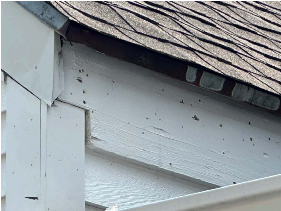
Image #24. WOOD SIDING AT FLAT ROOF AREA, SEPARATION OF ALUMINUM TRIM WORK, REUSE OF OLD ROOF COMPONENTS AT SHINGLE ROOF REAR ELEVATION
