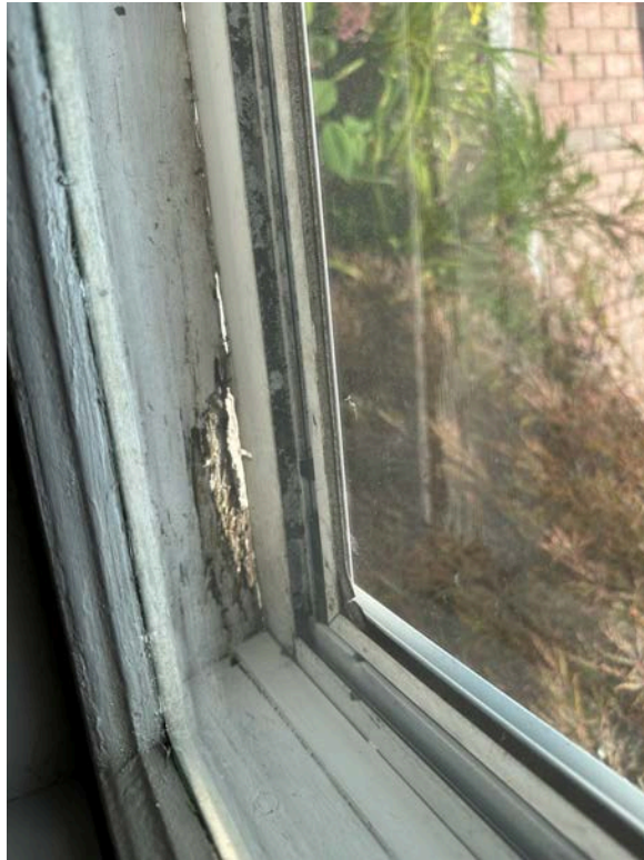
Image #49. ROTTEN WOOD FRAME, FROM INTERIOR FRONT ELEVATION
