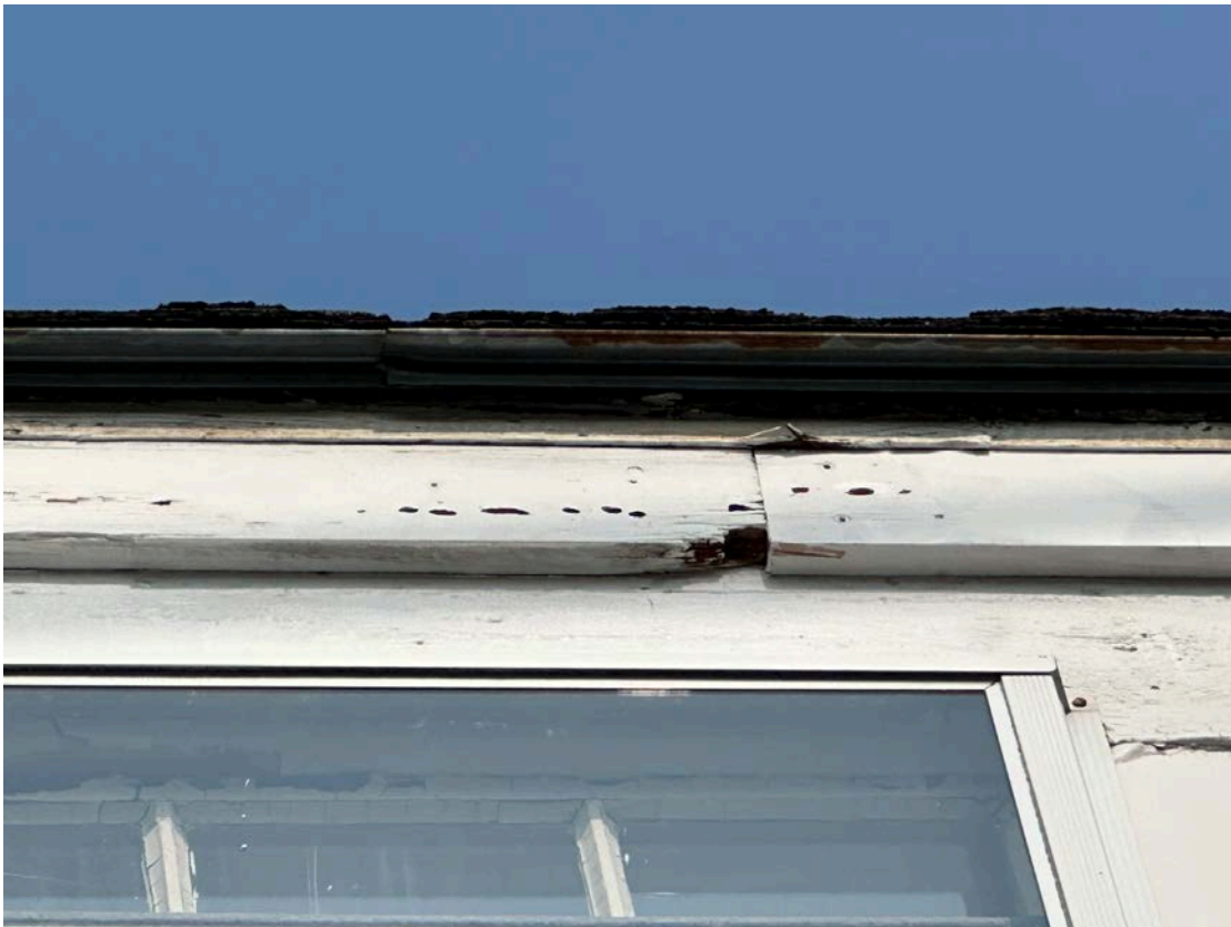
Image #31. DAMAGE TO TRIM AT ROOF LINE FRONT ELEVATION
