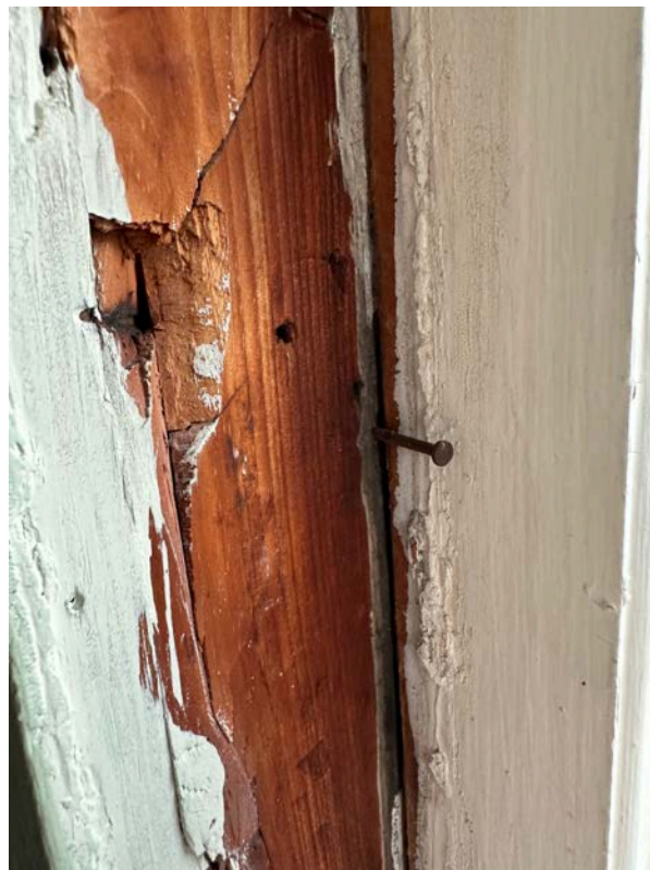
Image #60. MISSING TRIM AND MECHANISM, FROM INTERIOR FRONT ELEVATION
