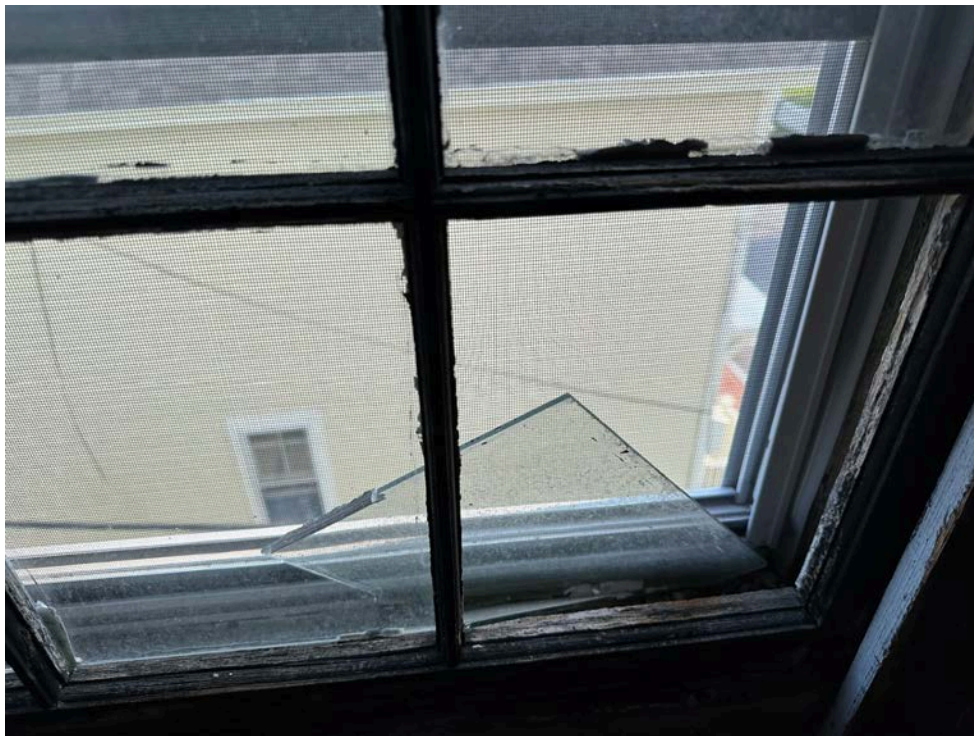
Image #38. BROKEN WINDOW PANES ATTIC FACING HOLMES COURT
