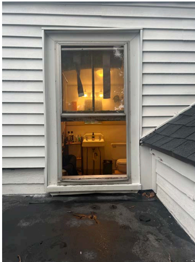
Image #10. LOCATION OF CASEMENT WINDOW (DOUBLE HUNG) REAR ELEVATION (OVER FLAT ROOF)
