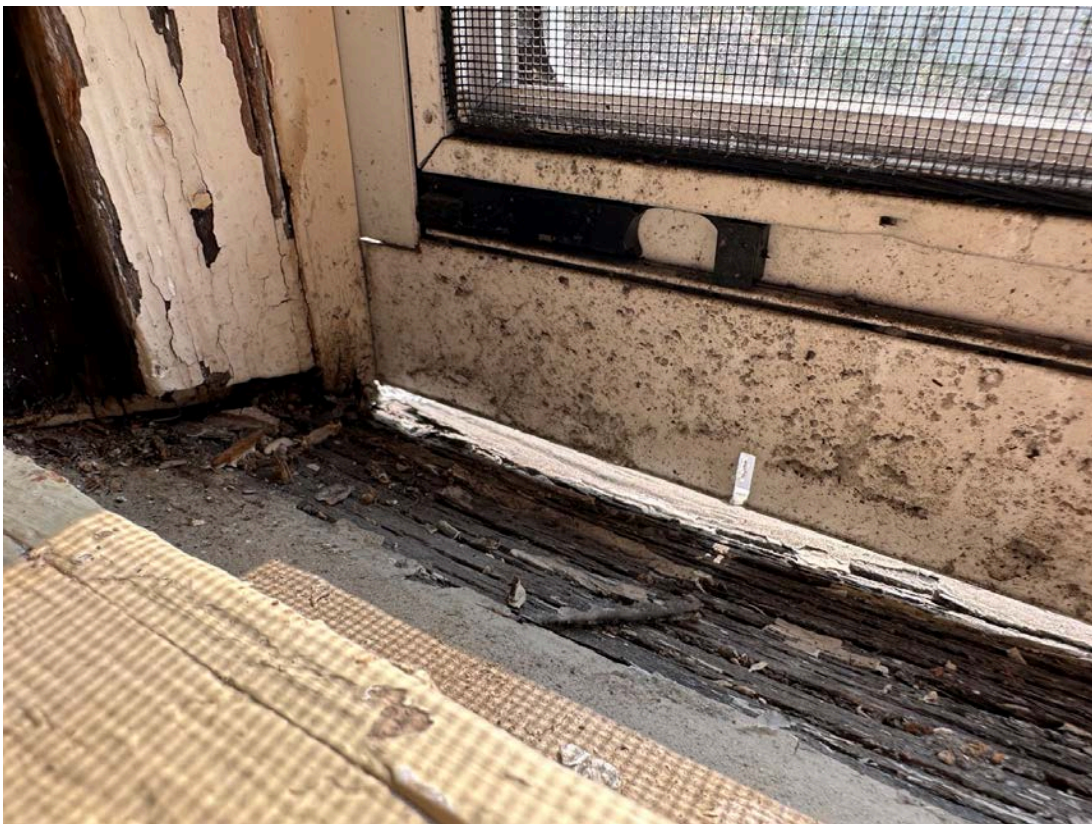
Image #58. ROTTEN SILL AND FRAME, FROM INTERIOR FRONT ELEVATION
