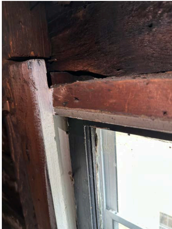
Image #66. ATTIC WINDOW, NAILED IN PLACE RIGHT ELEVATION
