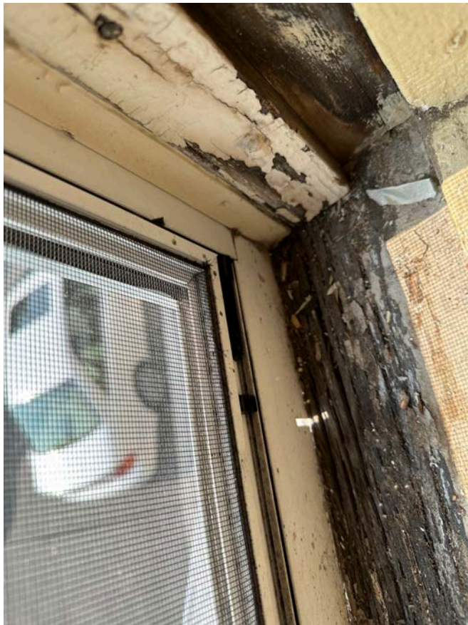
Image #57. ROTTEN WINDOW SILL AND FRAME, FROM INTERIOR FRONT ELEVATION
