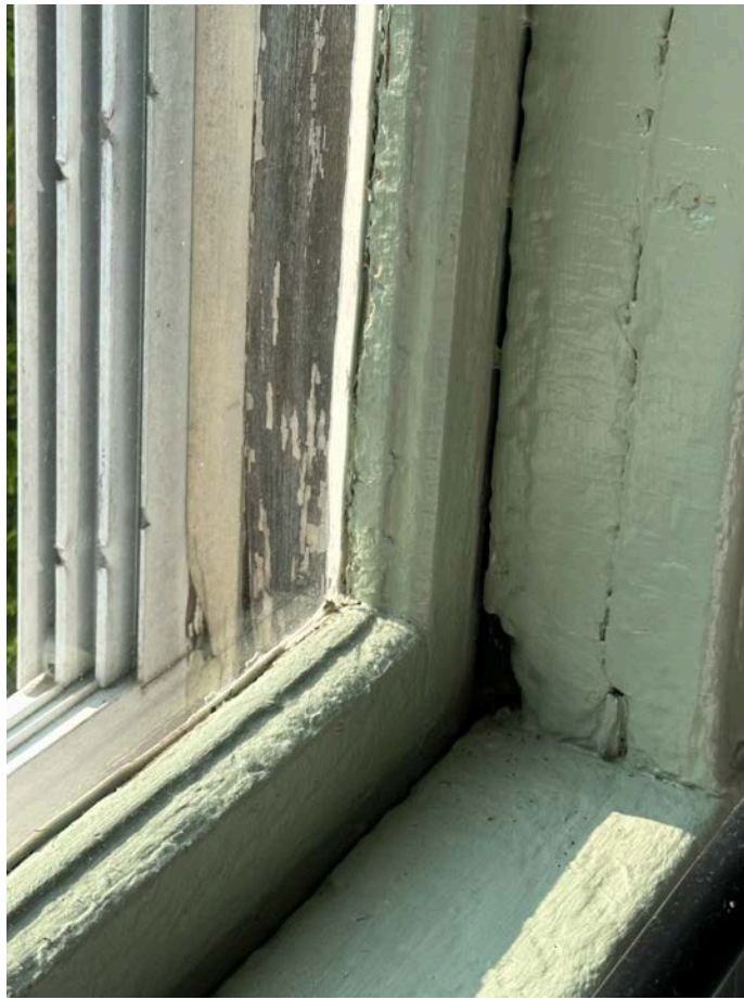
Image #53. ROTTEN WOOD FRAME, FROM INTERIOR FRONT ELEVATION
