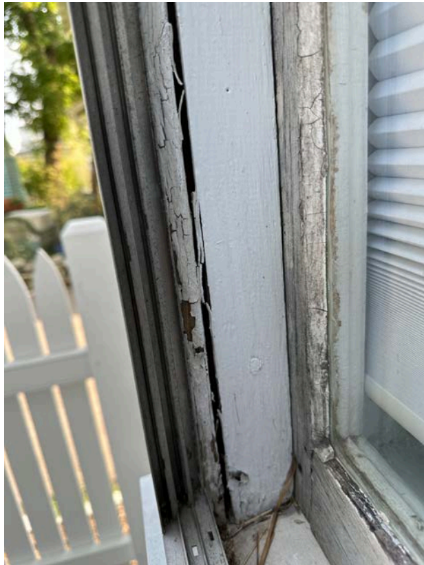
Image #40. WINDOW FRAME SEPARATION AND WATER DAMAGE REAR ELEVATION
