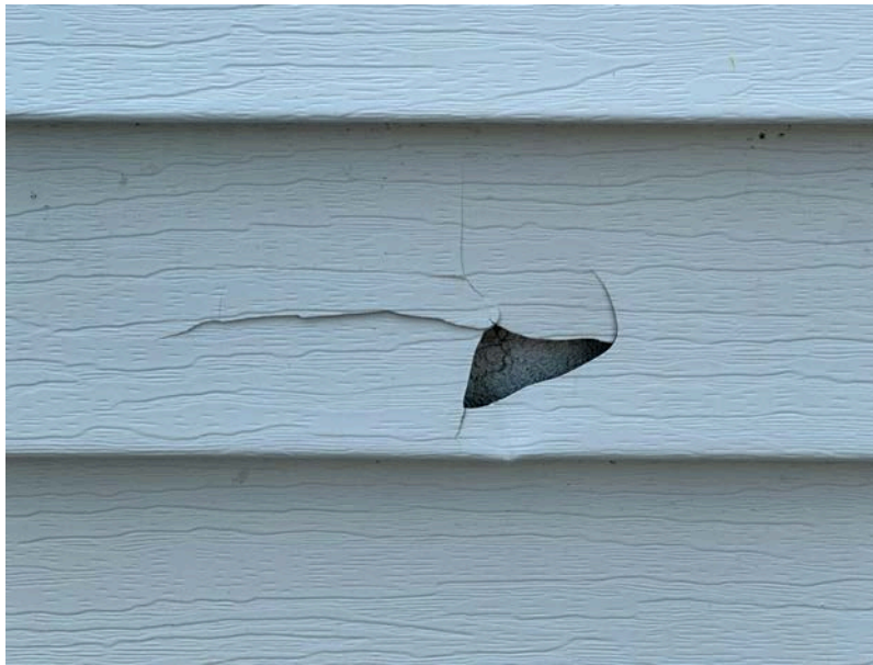
Image #19. DAMAGE TO VINYL SIDING REAR ELEVATION
