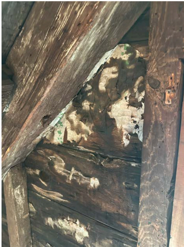
Image #65. FIRE DAMAGE ADJACENT TO ATTIC WINDOW RIGHT ELEVATION
