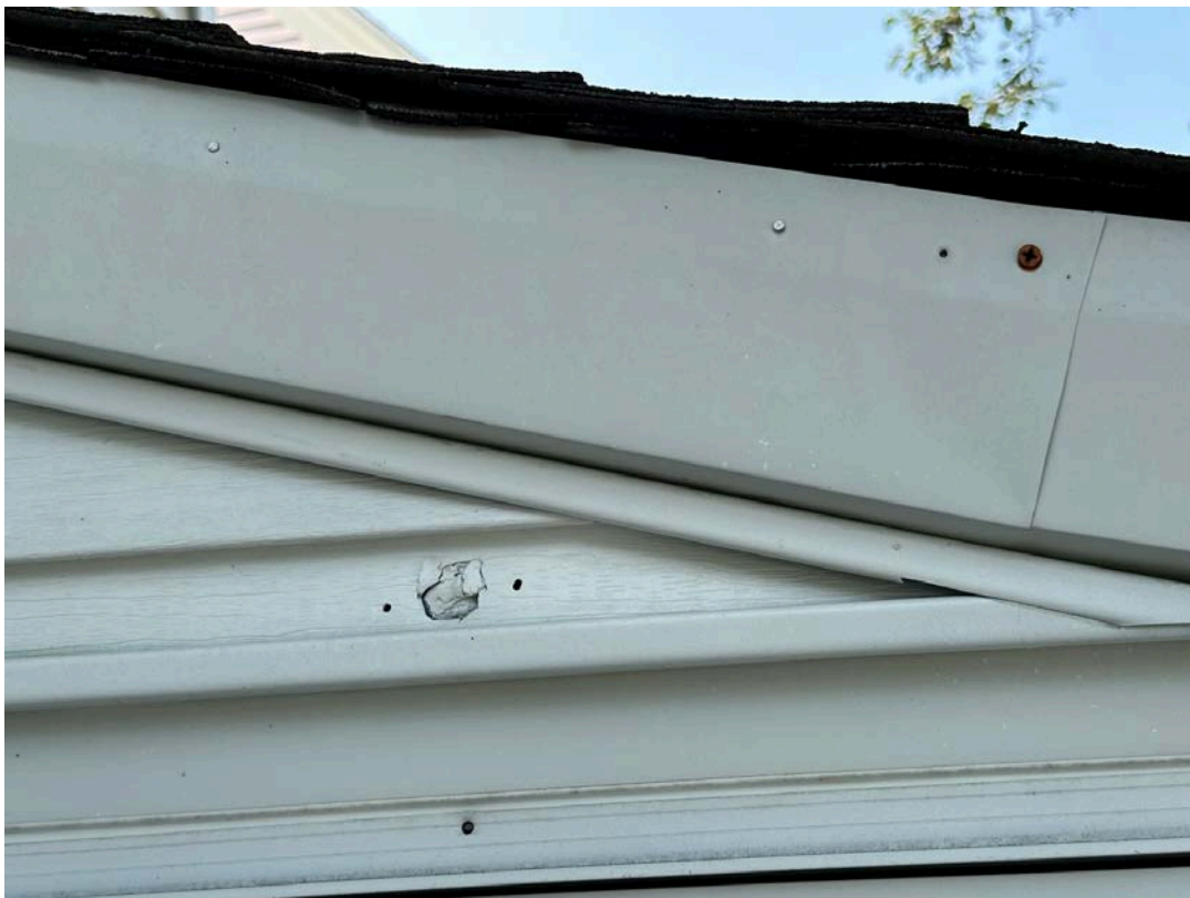
Image #26. DAMAGE TO VINYL SIDING REAR ELEVATION, PORCH
