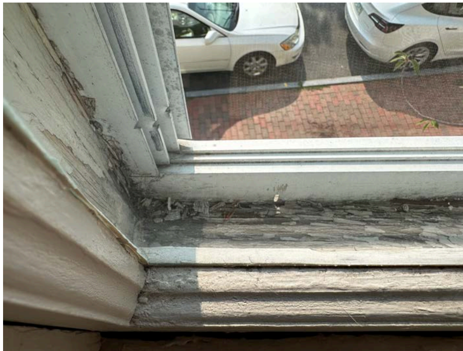
Image #56. ROTTEN WINDOW SILL, FROM INTERIOR FRONT ELEVATION
