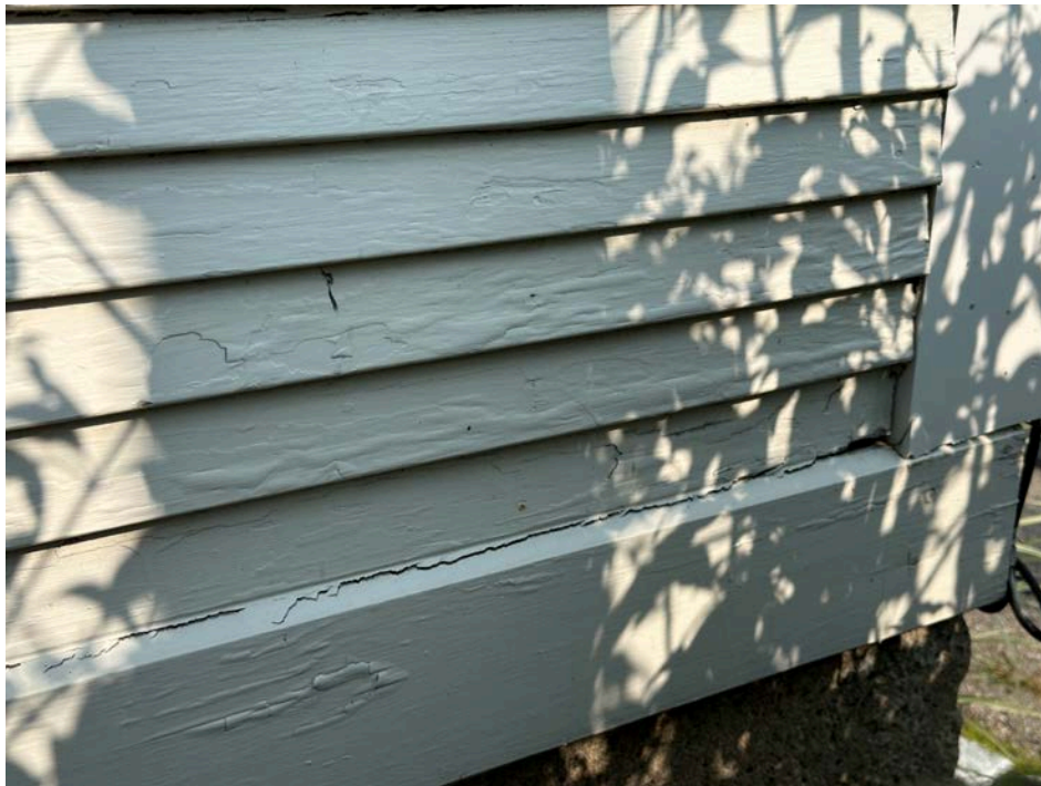
Image #20. WATER DAMAGE TO SIDING AND TRIM FRONT ELEVATION
