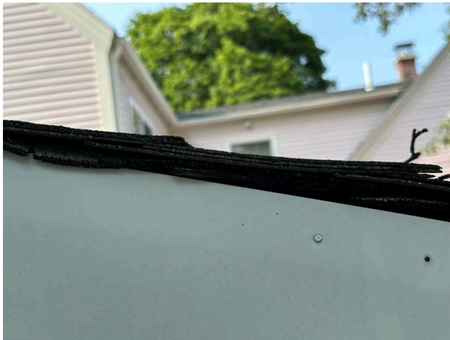
Image #30. INCOMPLETE INSTALLATION OF ROOF REAR ELEVATION, PORCH
