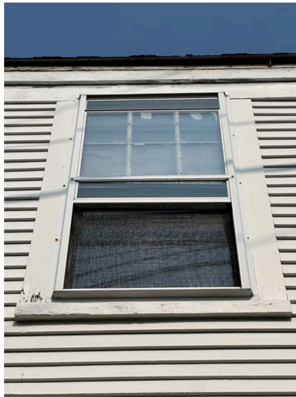
Image #36. WOOD ROT IN WINDOW TRIM; WOOD ROT IN UPPER TRIM FRONT ELEVATION
