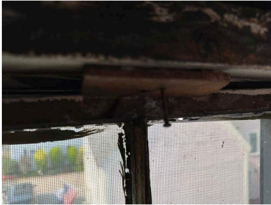
Image #63. ATTIC WINDOW MECHANISM MISSING, SECURED BY NAIL LEFT ELEVATION
