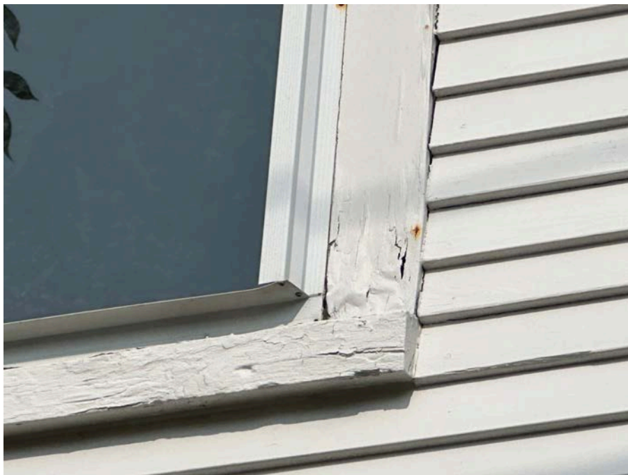
Image #34. WOOD ROT IN WINDOW TRIM FRONT ELEVATION
