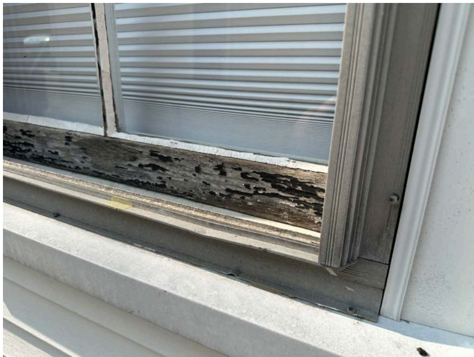
Image #42. STORM WINDOW, MISSING COMPONENTS REAR ELEVATION
