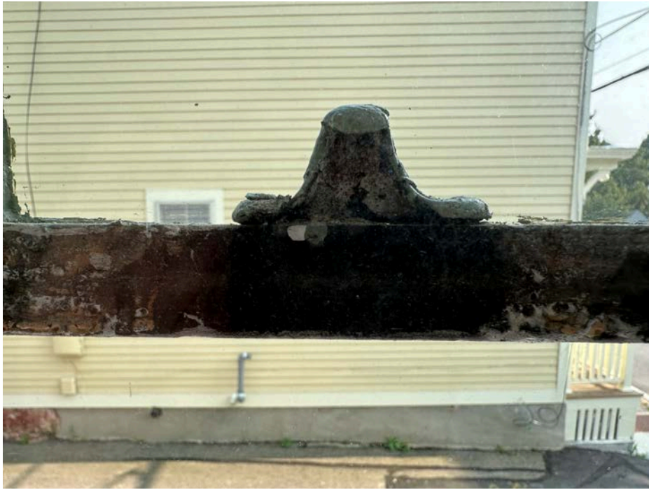
Image #51. ROTTEN WOOD FRAME, FROM INTERIOR RIGHT ELEVATION
