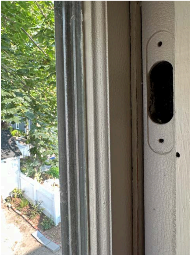
Image #55. MISSING WEIGHT SYSTEM, FROM INTERIOR REAR ELEVATION
