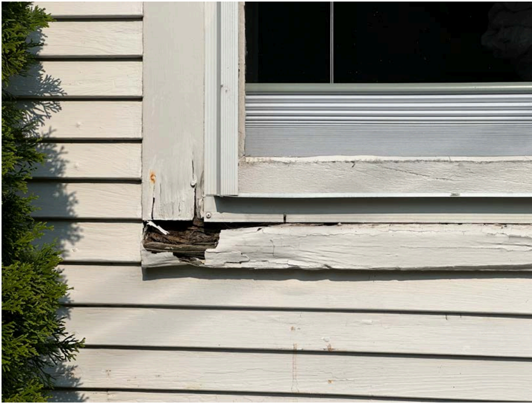
Image #35. WOOD ROT IN WINDOW SILL AND DAMAGED STORM WINDOW FRONT ELEVATION
