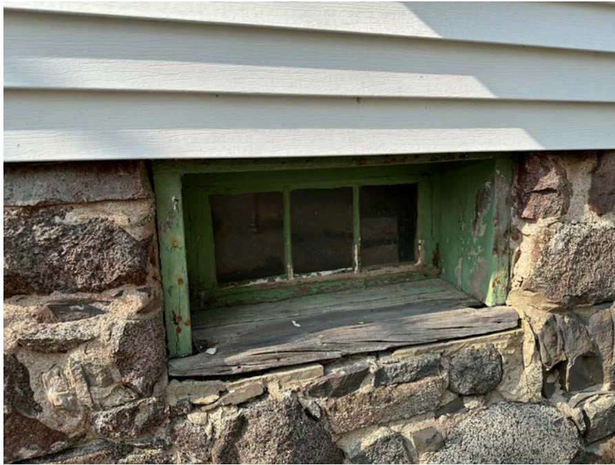
Image #13 BASEMENT WINDOW RIGHT ELEVATION, EXCLUDED
