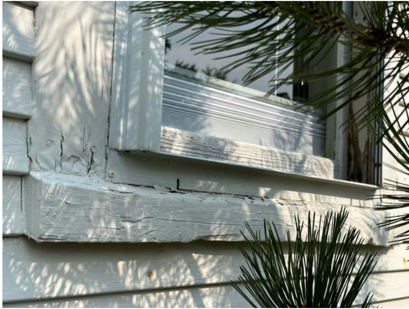
Image #37. WOOD ROT IN WINDOW SILL AND TRIM FRONT ELEVATION
