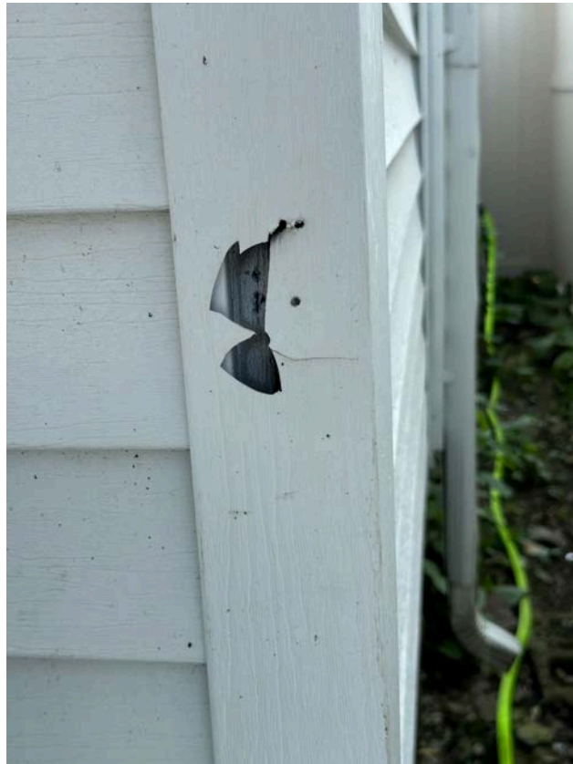
Image #22. DAMAGE TO VINYL TRIM REAR ELEVATION, PORCH
