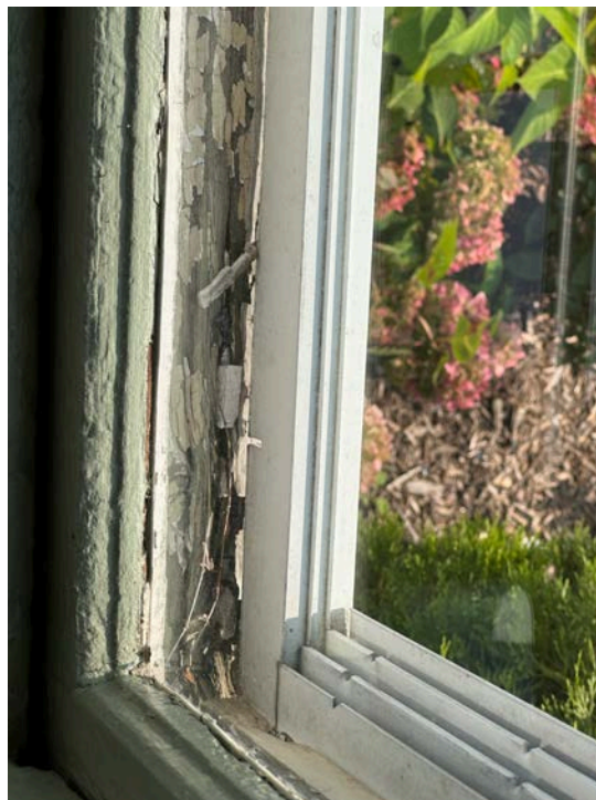
Image #54. ROTTEN WINDOW FRAME AND SEPARATION FROM STORM WINDOW, FROM INTERIOR FRONT ELEVATION
