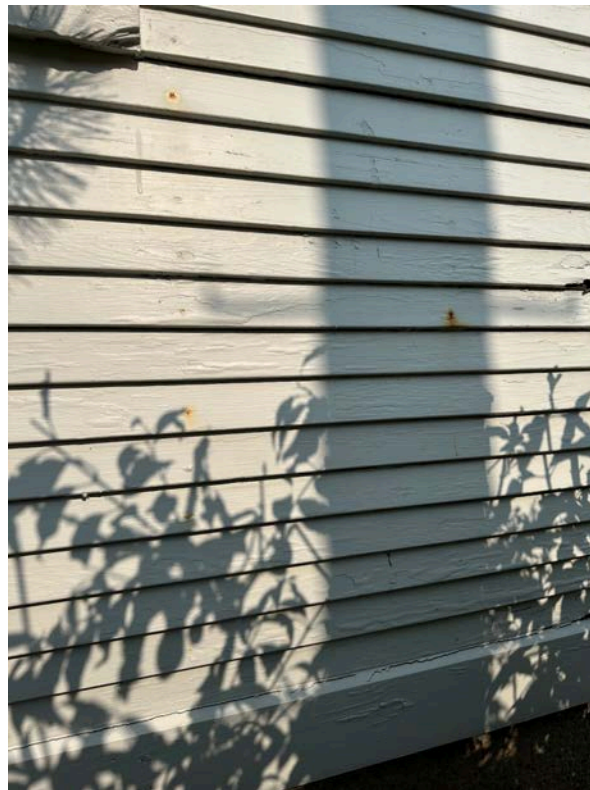
Image #18. WOOD ROT IN CEDAR SIDING AND TRIM FRONT ELEVATION
