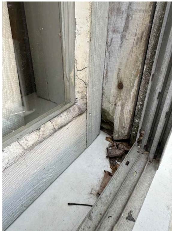
Image #44. ROTTEN WINDOW FRAME WITH WATER DAMAGE REAR ELEVATION, CENTER
