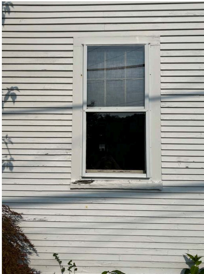
Image #33. ROTTEN FIRST FLOOR WINDOW SILL, DAMAGED STORM WINDOW, AND TRIM WORK FRONT ELEVATION
