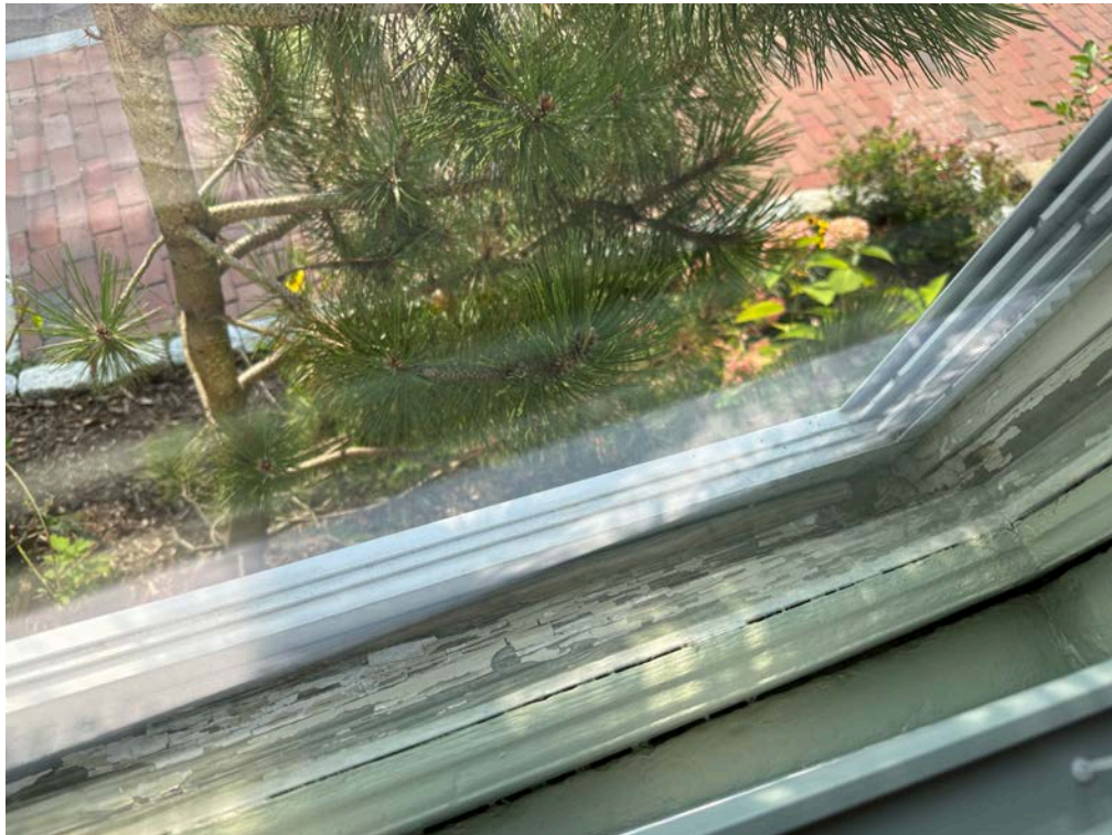
Image #52. ROTTEN WINDOW SILL, FROM INTERIOR FRONT ELEVATION
