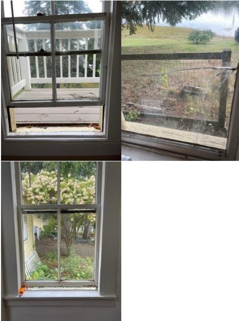
Various Samples of Damaged Windows (broken windows and rotted sashes)
