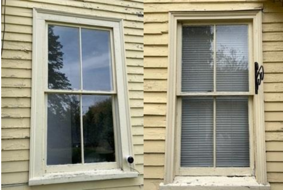
Closeup of Rebuilt Sills and Frames (note where sills were rebuilt at same 14 degree slope)
