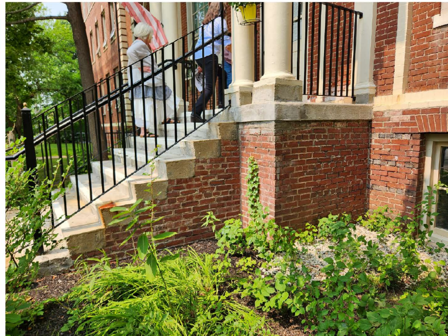
SOUTH ENTRY PRIOR REPAIR MASONRY FAILURE
