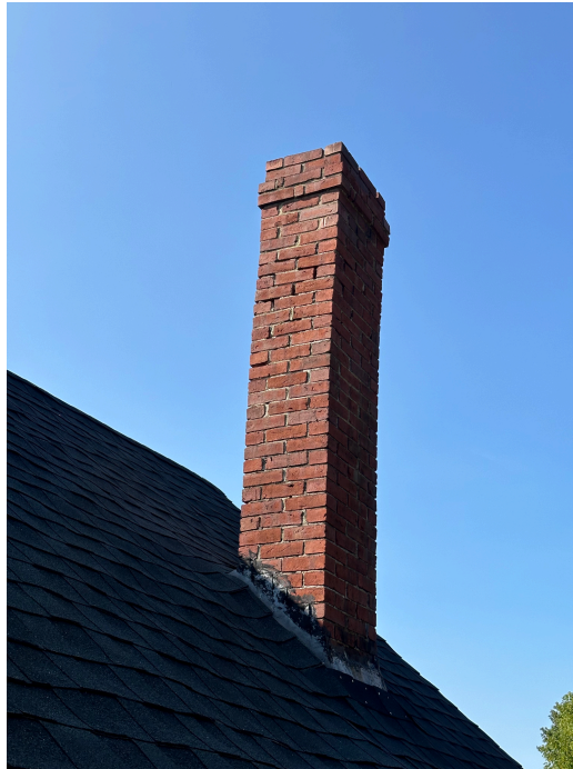
Image #1. TALLER CHIMNEY AT LEFT ELEVATION, photo taken from rear In use, to be repointed with historic mortar of matching color
