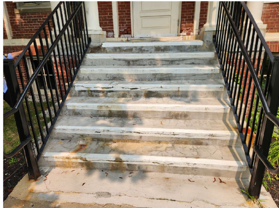
SOUTH ENTRY DAMAGED STAIRS
