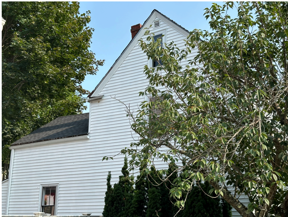
Image #4. EXISTING LEFT ELEVATION VIEW FROM MARCY STREET, taller chimney (to remain) visible
