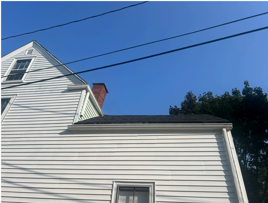
Image #6. EXISTING RIGHT ELEVATION VIEW FROM HOLMES COURT, shorter chimney (to be removed) visible
