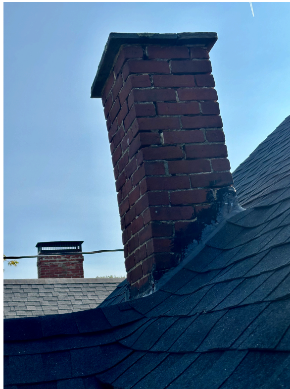
Image #2. SHORTER CHIMNEY AT RIGHT ELEVATION, photo taken from rear Disused, to be removed
