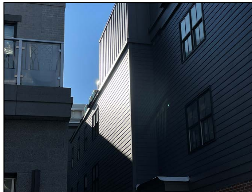
PERSPECTIVE OF SERVICE DECK FROM DEER STREET (SCREENING HAS NOT BEEN INSTALLED YET)
