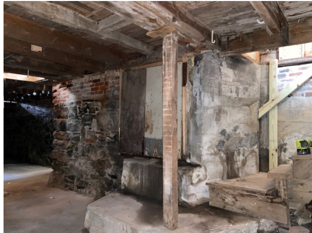
16-Timber post supporting decayed joist
