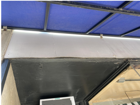
2 - WATER INFILTRATION AT ENTRY AREA AT EYELOOK OPTICAL
