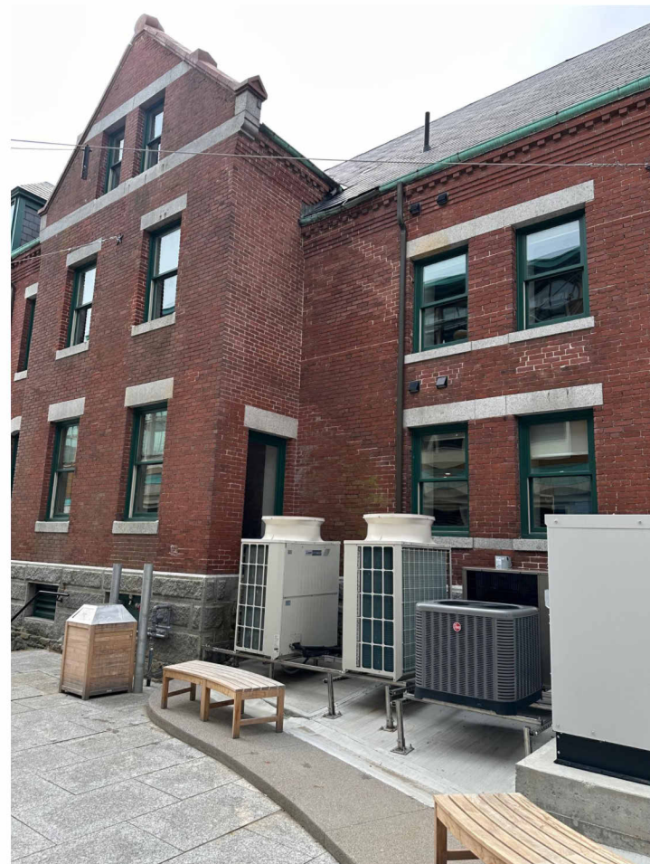
EXISTING COMPRESSOR TO BE COVERED
