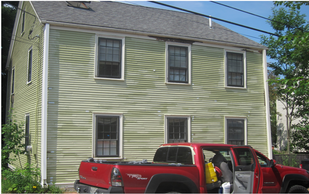
Front of House with rotting gutters, trimboard, siding and cornerboards
