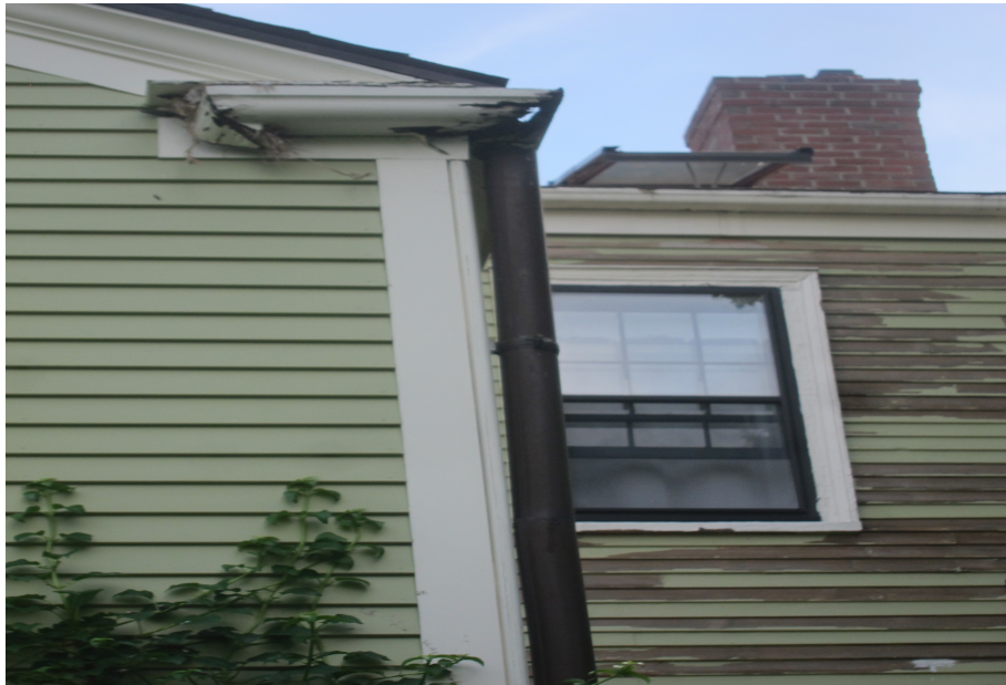
Rot on Back Addition Gutters and Main House siding, trim and window mouldings
