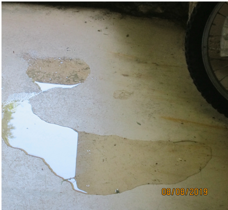
Illustration 2: Water in Basement Under the Main House
