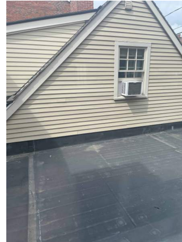
ADJACENT PROPERTY - 100 STATE STREET UNPERMITTED/NON-CONFORMING WINDOW
