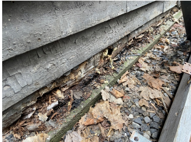
6-Wood decay along west side
