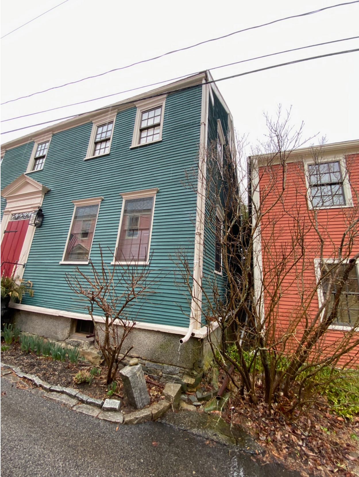
Downspout disconnected from gutter – requires weekly repair
