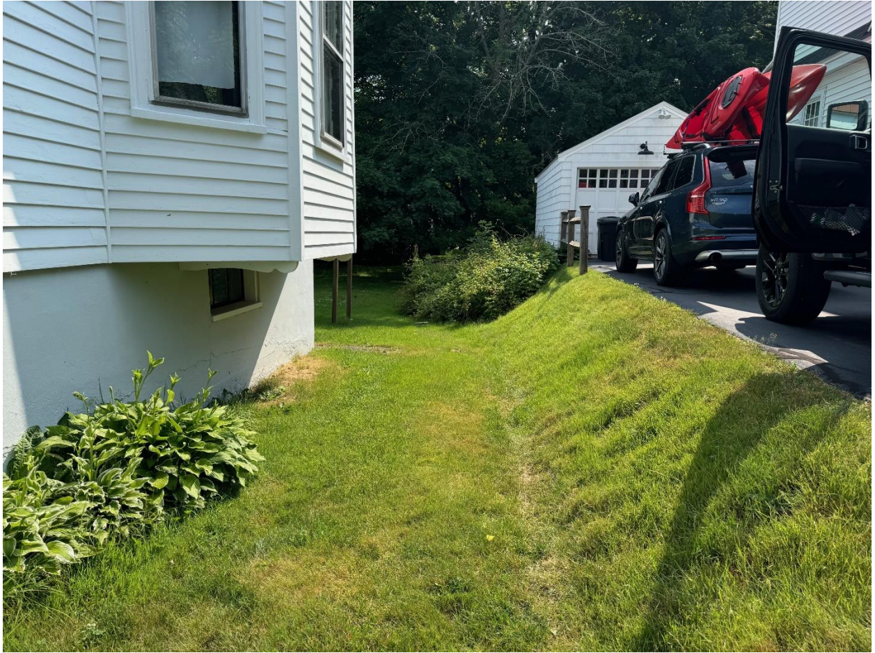
Exhibit – View of grade change/slope between 189 and 199 Wibird St.
