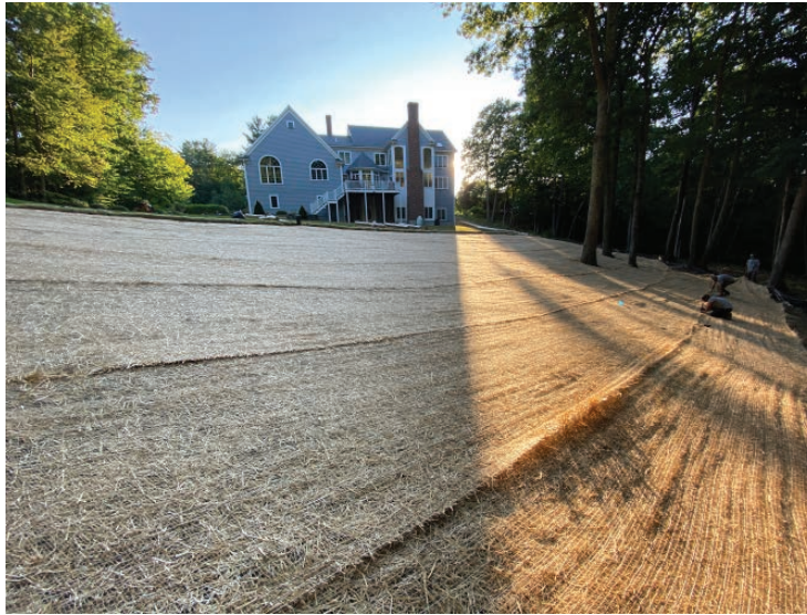
3. Covered exposed loam with straw erosion control blanket: BioNet S75BN and staple into existing slope
