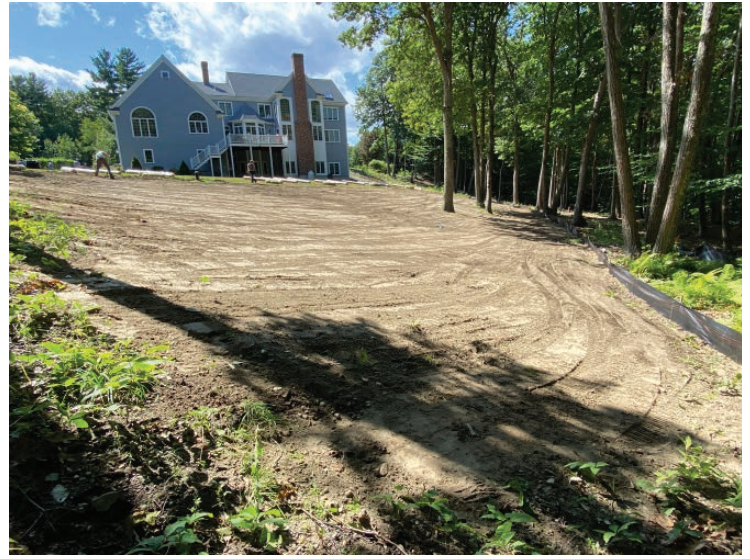
2. After installation of sediment control, we mechanically mowed area and seeded with New England Conservation and Wildlife Seed Mix
