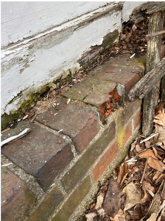
FOUNDATION SHELF AND ROT FROM STANDING WATER
