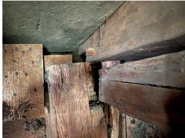
24-Vertical split at corner post
