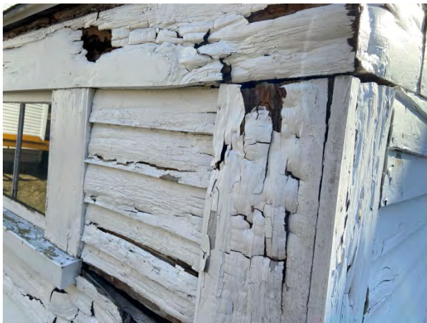
15-Barn decay damage
