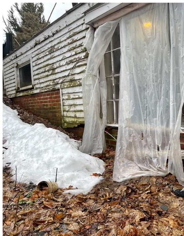
TYPICAL SIDING ROT AND FOUNDATION DAMAGE
