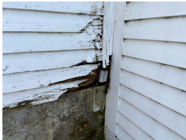
16-Barn decay damage
