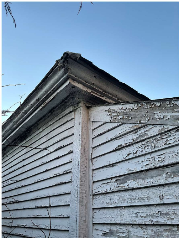
TYPICAL SIDING ROT
