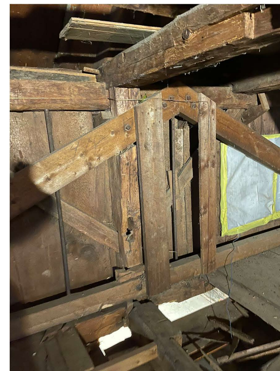
OLDER FRAMING MEMBERS HAVE BEEN MODIFIED, REMOVED, OR RELOCATED. (SECOND FLOOR OF CARRIAGE HOUSE)
