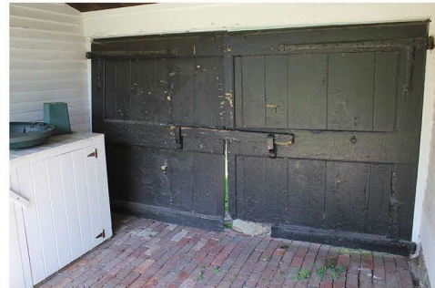
ORIGINAL HISTORIC DOORS TO BE REMOVED, RESTORED, AND REINSTALLED ON NEW CONNECTOR CONSTRUCTION
