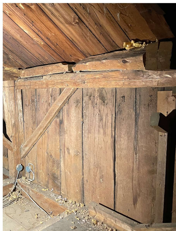
OLDER FRAMING MEMBERS HAVE BEEN MODIFIED, REMOVED, OR RELOCATED. (SECOND FLOOR OF CARRIAGE HOUSE)
