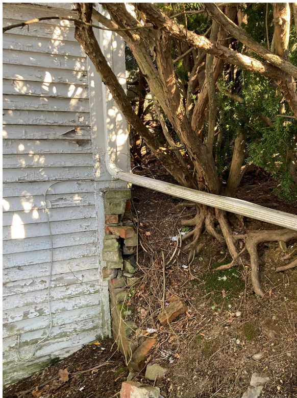
CRUMBLING FOUNDATION LACKING POSITIVE DRAINAGE
