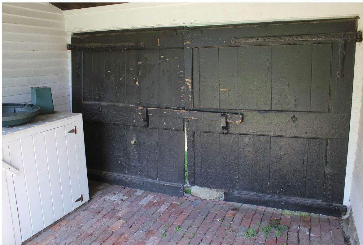
POSSIBLE HISTORIC DOOR WITH HISTORIC HINGES
