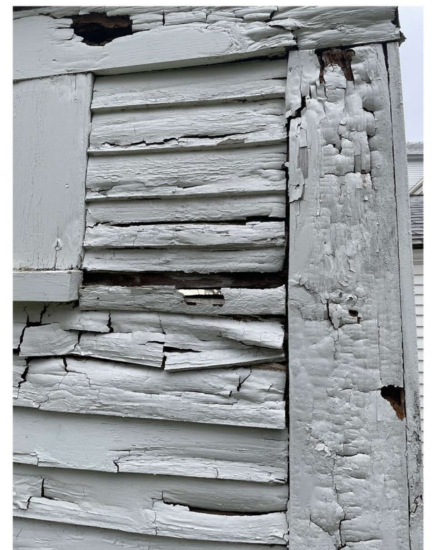
SIDING ROT AND INSUFFICIENT FLASHING
