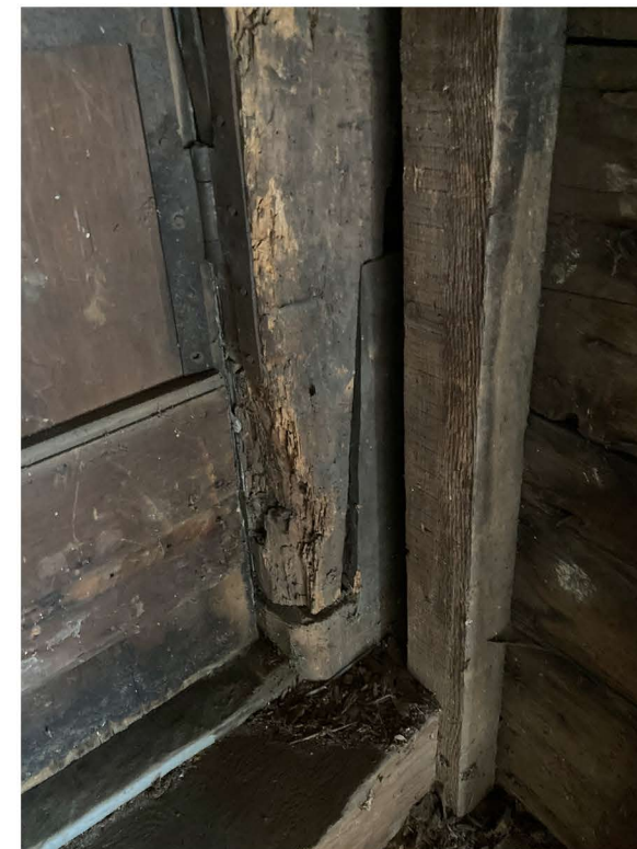
TYPICAL HALF LAP POST ROT REPAIR SEEN THROUGHOUT CONNECTOR
