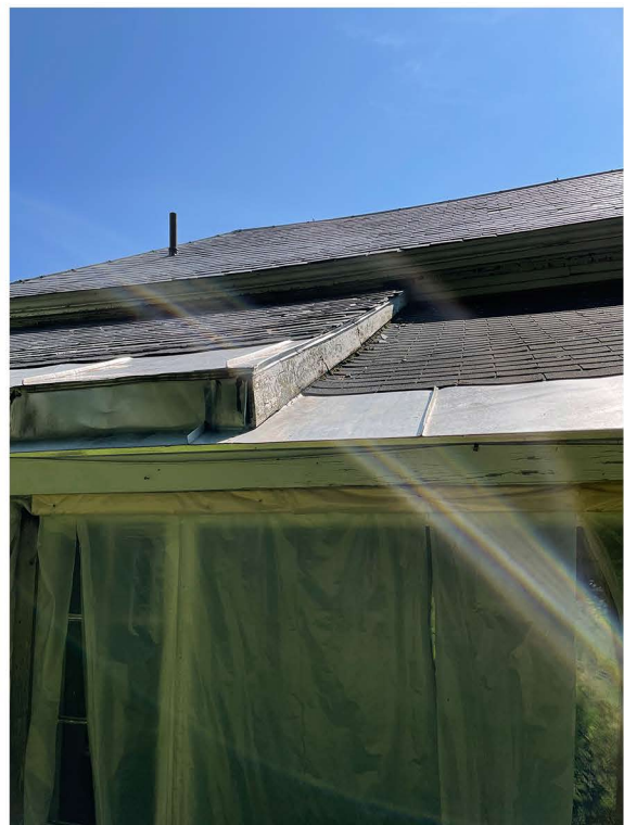
INSUFFICIENT ROOF FLASHING
