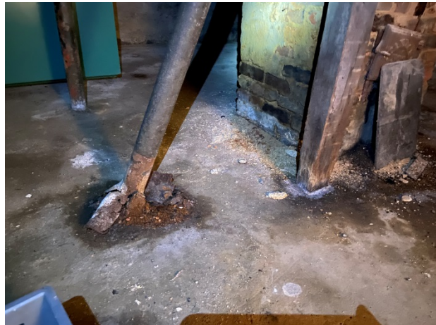
28-Failed column and wood post
