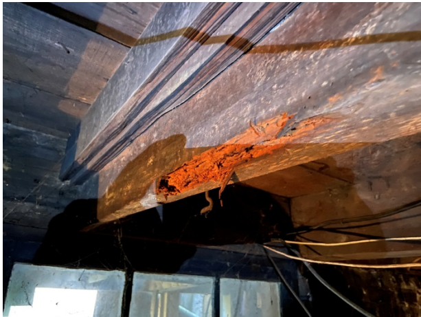
27-Decayed floor joist
