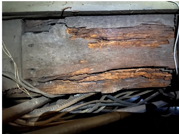
26-Decayed floor joist
