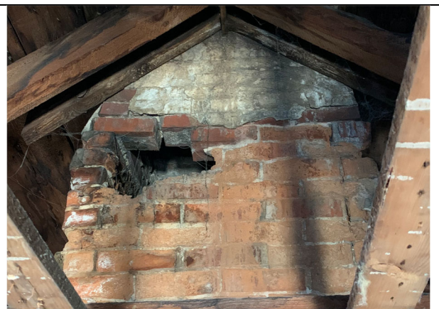
Hole in chimney, brick in poor condition
