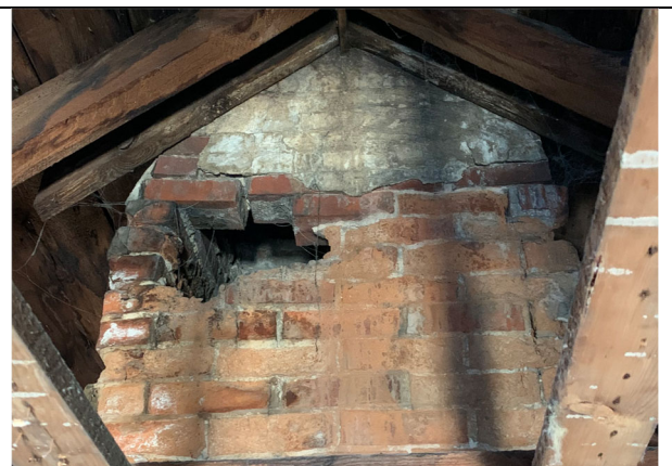
Hole in chimney, brick in poor condition
