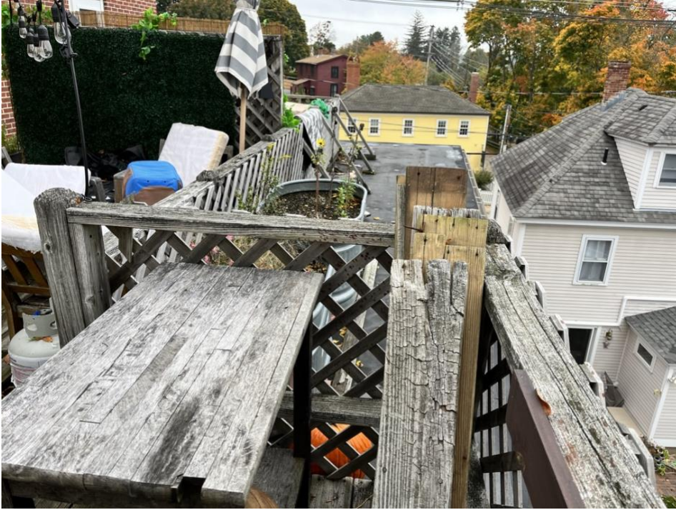
Figure 7. Rooftop as seen facing Maplewood and showing existing railing with lattice and propped vs. secured. Also showing exposed EPDM to edge.
