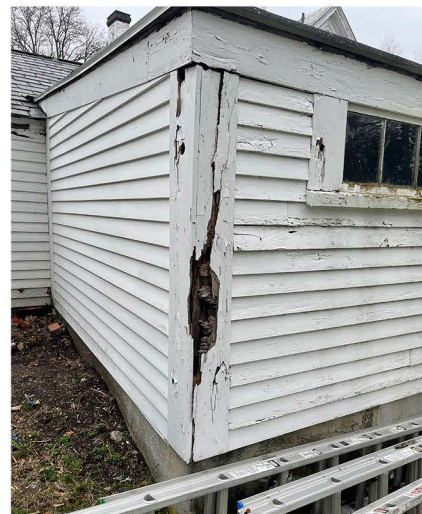
CORNER BOARD ROT
