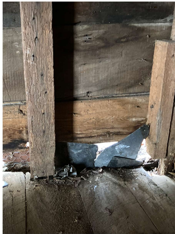
COMPROMISED STRUCTURE AT BASE
