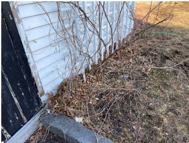
9-Siding extending below grade
