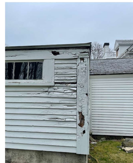
SIDING / CORNER BOARD ROT
