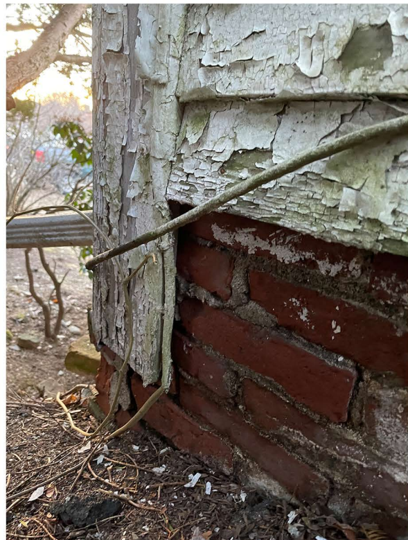
ROT FROM STANDING WATER
