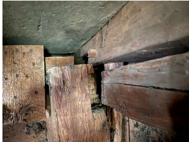
24-Vertical split at corner post
