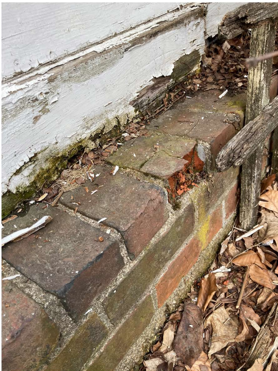
FOUNDATION SHELF AND ROT FROM STANDING WATER
