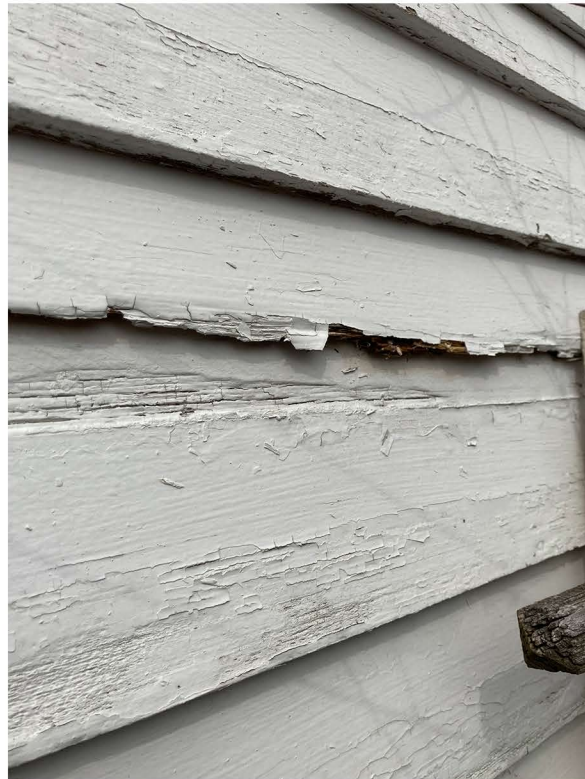
TYPICAL SIDING ROT
