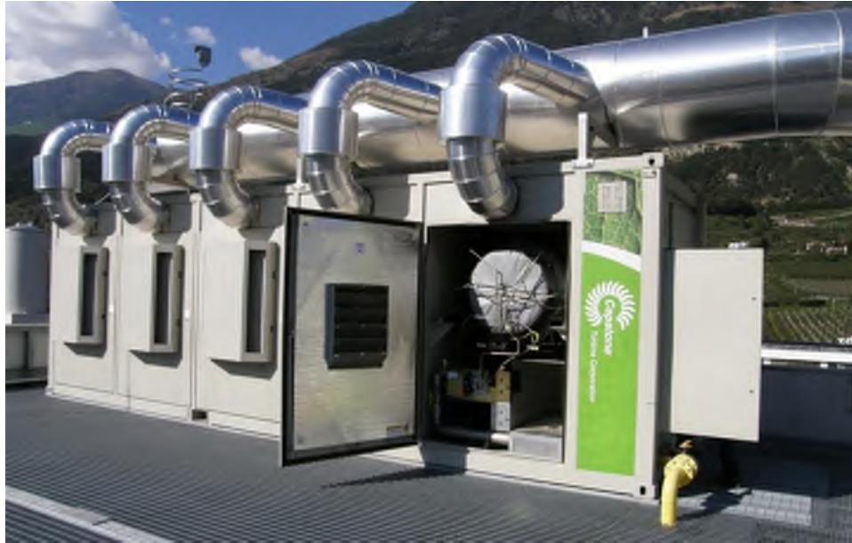
Figure 3-7. Capstone C1000, 1000 kW microturbine package with integrated exhaust manifold Sheboygan Regional WWTF, Wisconsin.
