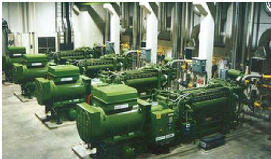
Figure 3-6. IC engine cogeneration system at Annacis Island WWTF in Vancouver, British Columbia
