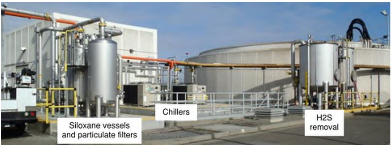
Figure 3-2. Gas conditioning system at the Santa Rosa Laguna Treatment Plant, including hydrogen sulfide removal vessels, siloxane removal vessels, and chillers
