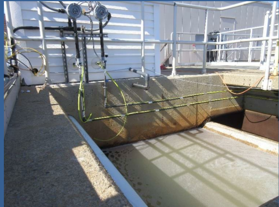
Chlorine Contact Tanks
