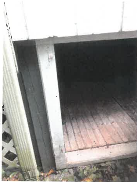
No foundation under bathroom
