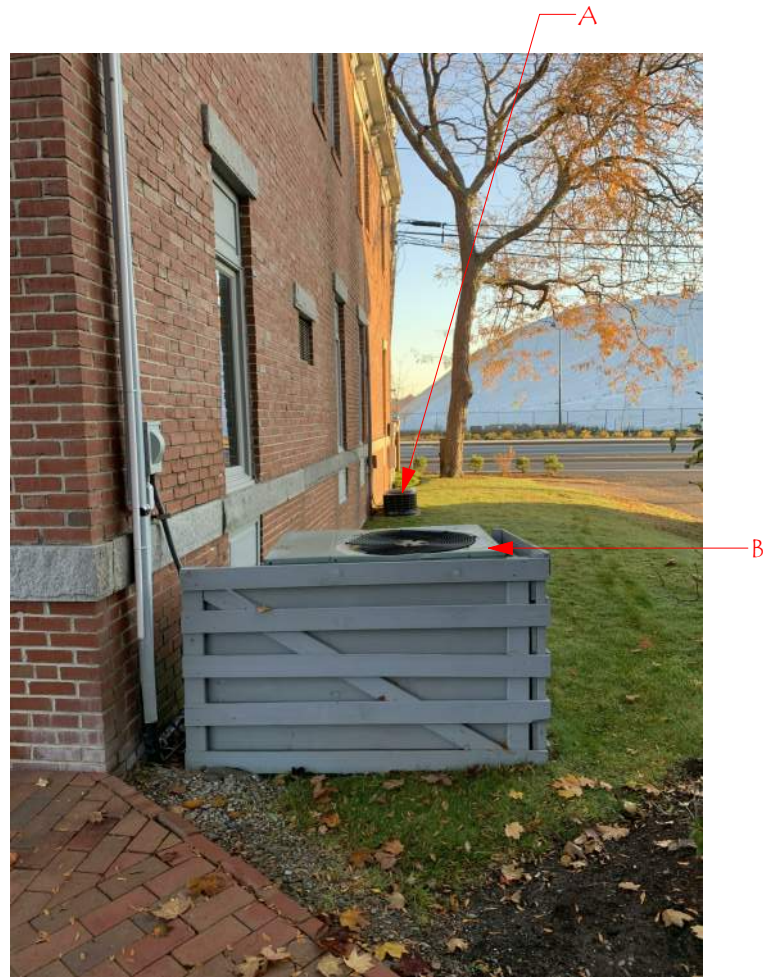
EXISTING/CURRENT CONDENSER LOCATIONS TO BE POSSIBLY REPLACED, AND SCREENED IN KIND.
