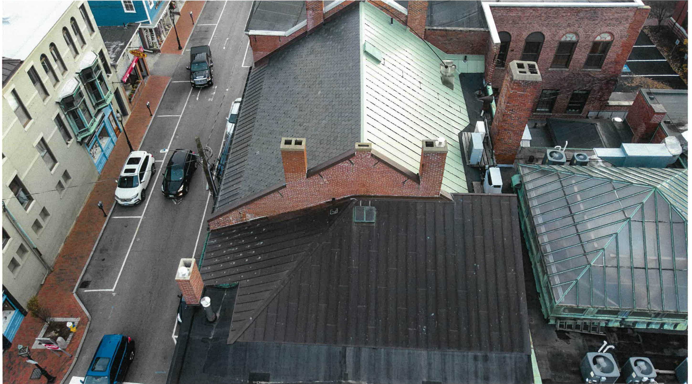
Proposed Upblast Fan installed on rear metal roof (not visible from public way)
