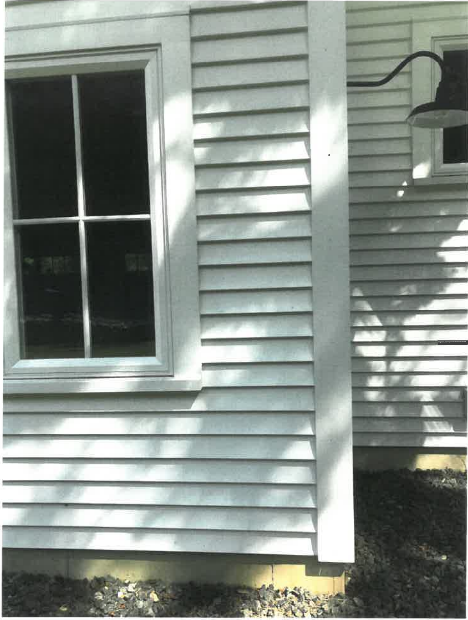
Window and Corner Trim 4 Lydia Lane-Closeup
