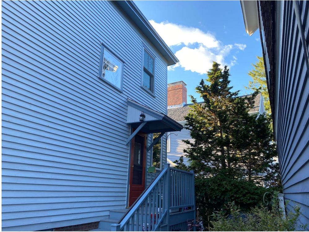
Condensers hidden by fence, and again by deck.
