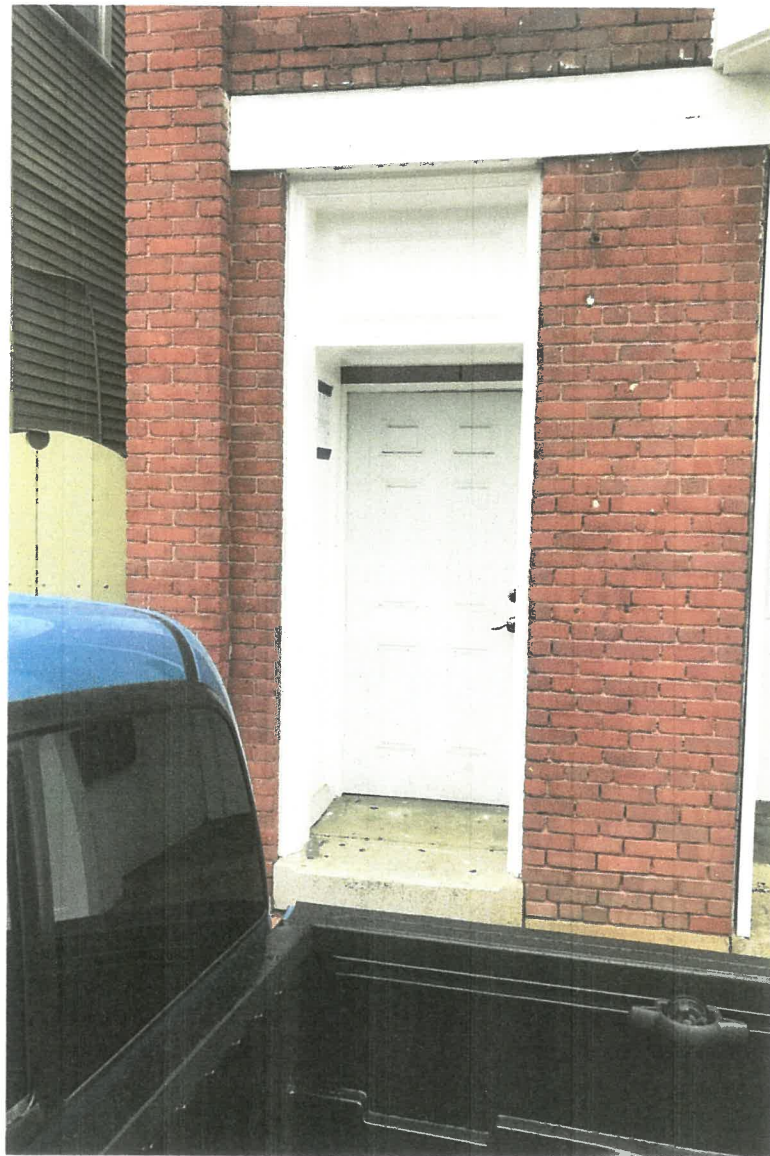
Door to Be Replaced
