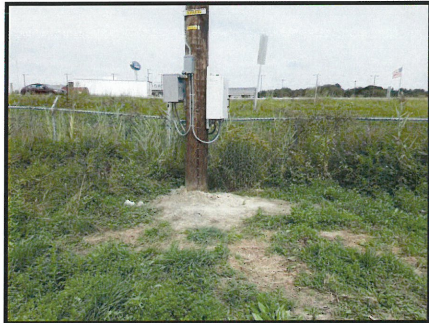
Photo 4. Previously disturbed area at new utility pole and SCADA Mate installation located within wetland PW1, facing east toward Route 16/Route 4 (Spaulding Turnpike).
