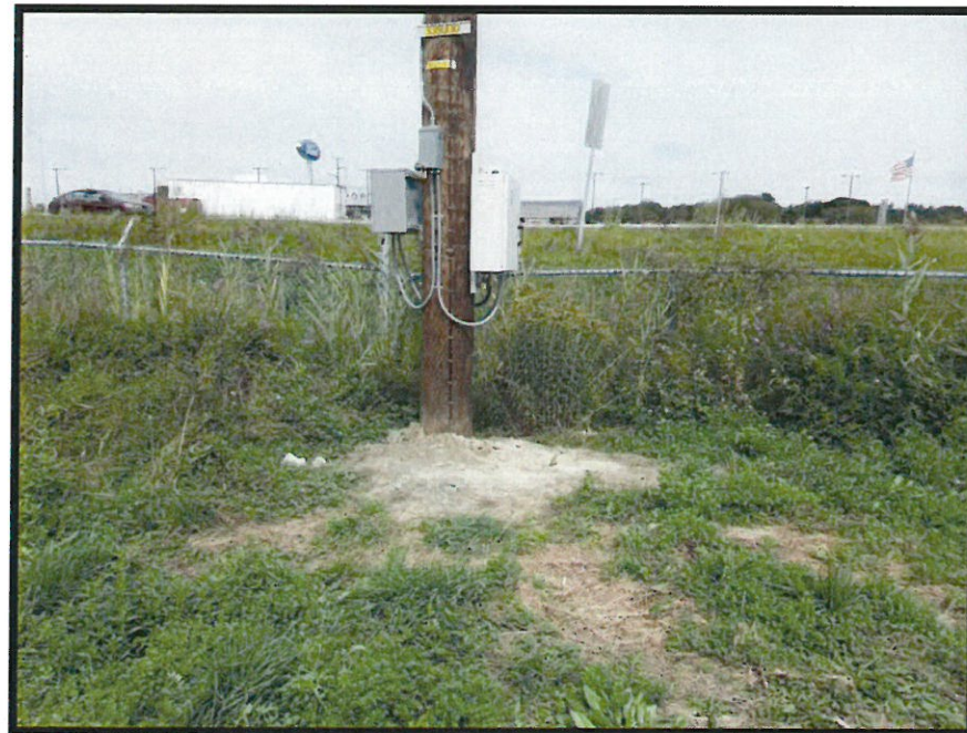
Photo 4. Previously disturbed area at new utility pole and SCADA Mate installation located within wetland PW1, facing east toward Route 16/Route 4 (Spaulding Turnpike)
