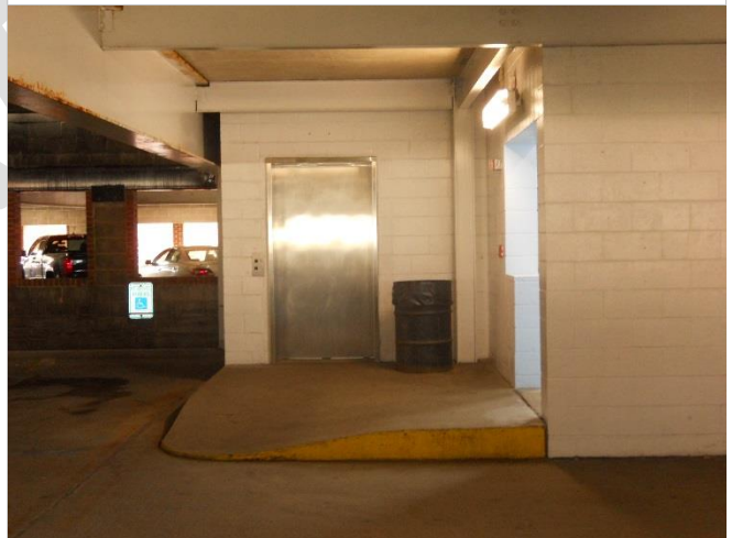
Photo 32 – Level 3 elevator stair lobby at stair #2. Note non-standard ADA curb drop .
