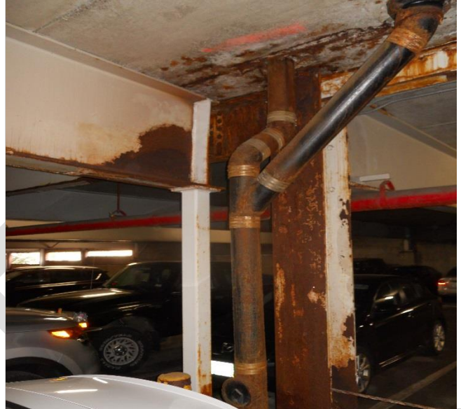
Photo 13 – Level 1 – Tube column support provided below beam due to sectional loss on steel girder.
