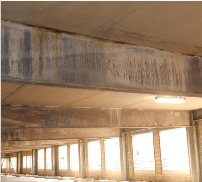
Photo 27 – Structural framing in garage expansion area (1999). Note straining and spotted rust on framing.
