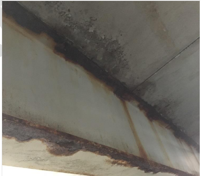
Photo 24 – View of corrosion on structural framing below deteriorated floor slab area.
