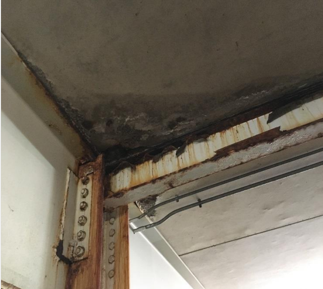
Photo 17 – Level 2 Floor slab deterioration and severe corrosion on structural framing.
