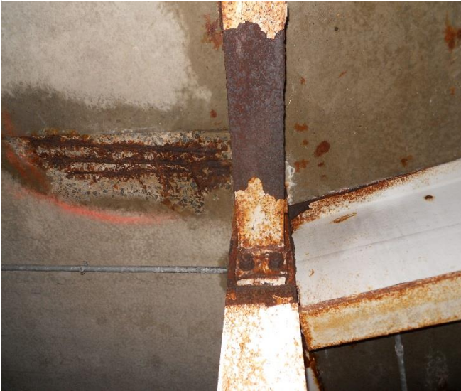
Photo 14 – Level 2 floor underside deterioration and staining on the precast filigree planks. Note corrosion damage to supporting beam.
