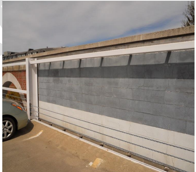
Photo 7 – North elevation interior view of façade CMU wall. Note progressive cracking on masonry block.
