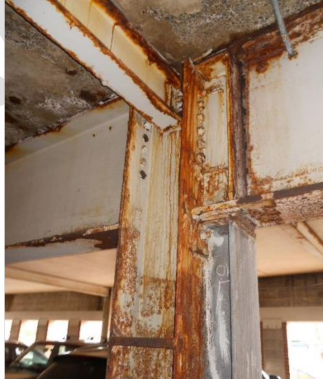
Photo 11 – Structural framing column and beam corrosion at east end of grade level 1. Note deterioration and staining on floor slab above.
