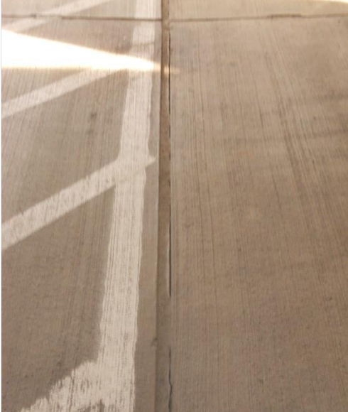
Photo 29 – Garage expansion area. View of typical joint sealant adhesion failures.
