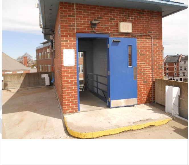
Photo 34 – Stair #3 raised walk at doorway. Note deterioration and separation of walk from floor slab.
