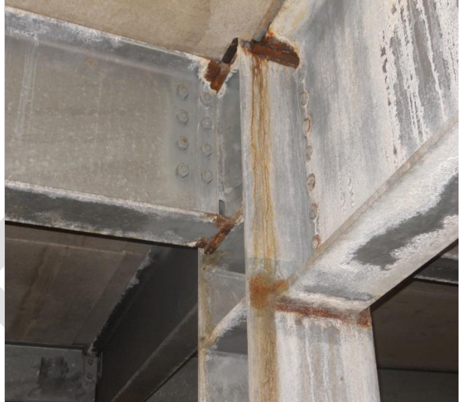
Photo 30 – Garage expansion area. Corrosion on weldments. Sealant failures noted above framing line.
