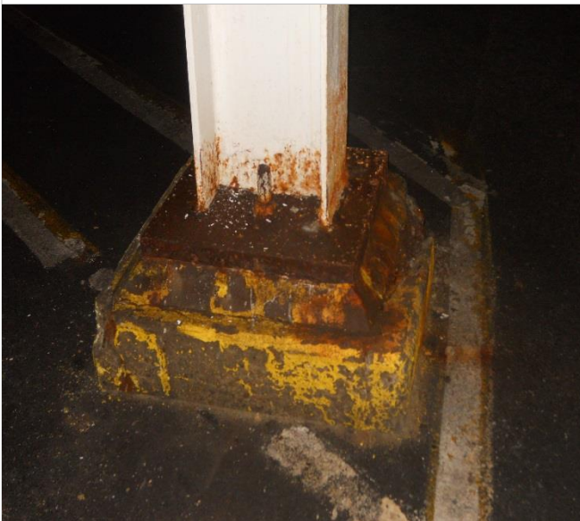
Photo 15 – level 1 – Corrosion on column base plate and deterioration of concrete pier.
