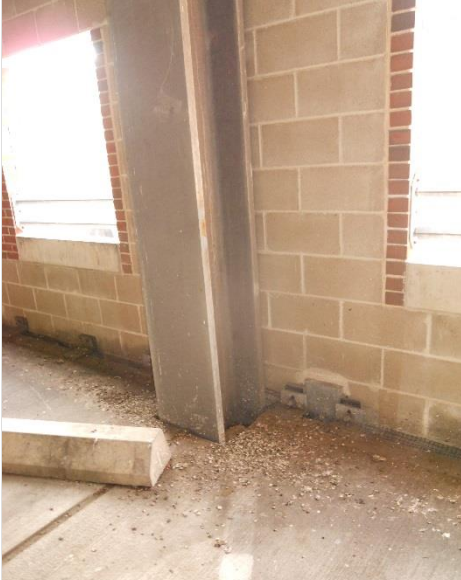
Photo 33 – Bird roosting problem in garage expansion area along south elevation.
