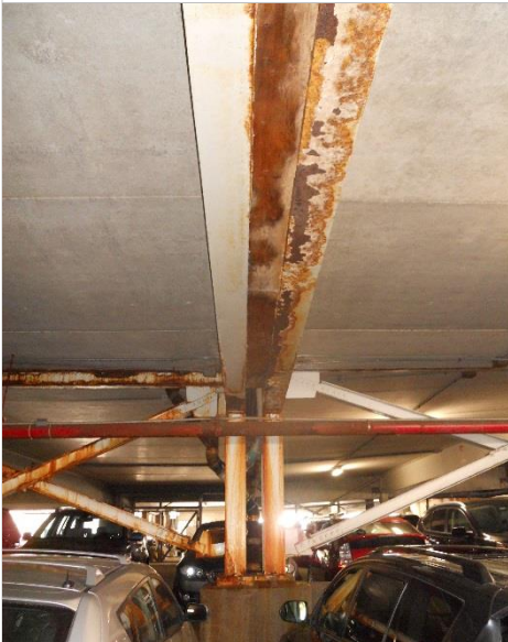
Photo 19 – Level 2 - underside framing corrosion along expansion joint line. Note corrosion on FP line.
