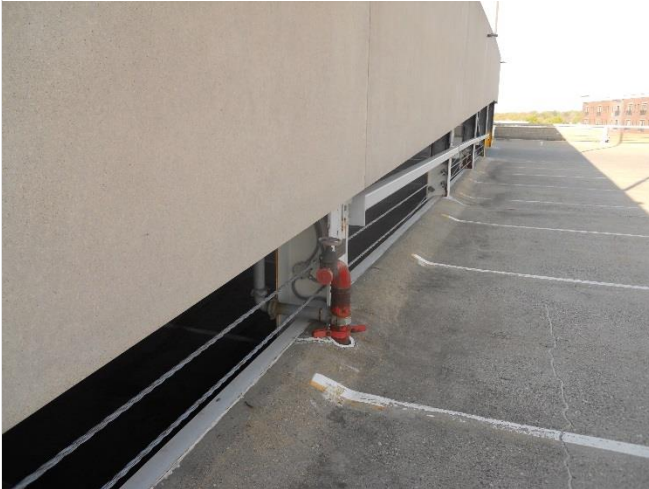
Photo 31 – Level 4 barrier guard railing. Note size of openness between cable strands.
