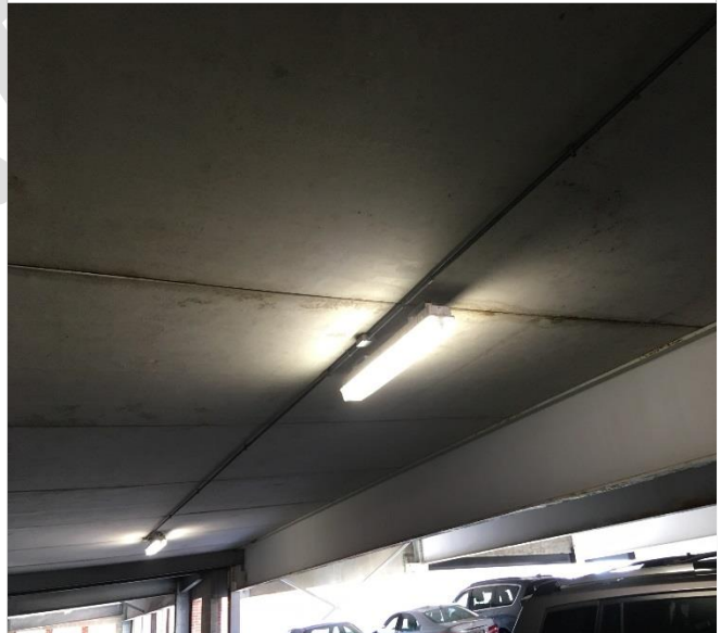
Photo 40 – General floor lighting with strip fluorescent fixtures.
