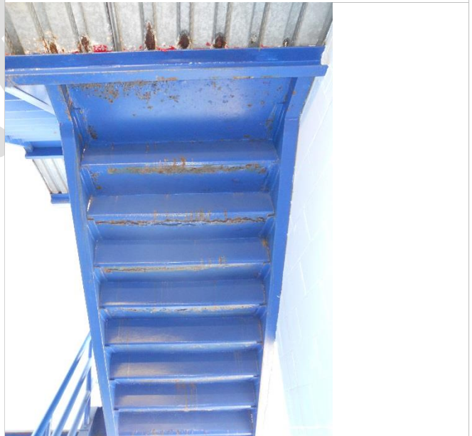
Photo 36 – Stair #1 corrosion damage to stair step pans.
