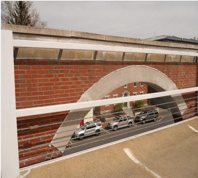
Photo 8 – North elevation interior view of façade masonry. Note protective netting applied to deteriorating masonry.
