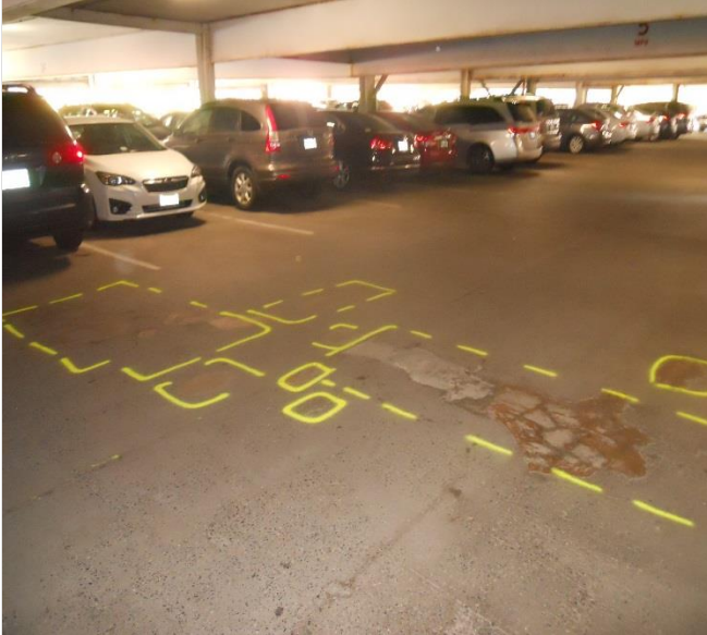
Photo 23 – Level 3 painted outline of deterioration formations above structural framing.
