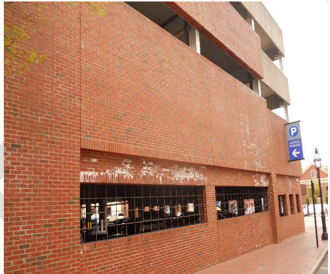
Photo 1 – View of façade northwest corner. Note staining on masonry veneer.
