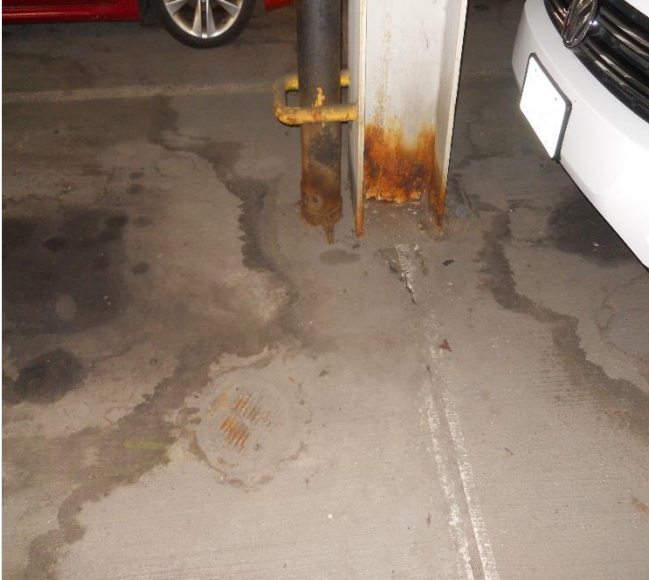
Photo 25 – Level 3 floor drain plugged with debris. Note water staining and corrosion around column and drain line.
