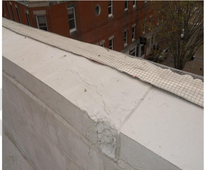
Photo 9 – deteriorated capstones on level 5 barrier wall. Note debris netting applied to top of wall as a precautionary measure.
