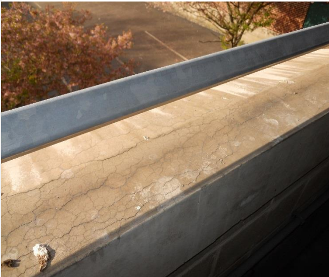
Photo 12 – Barrier wall capstone showing progressive pattern cracking.
