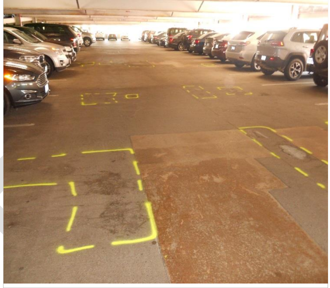
Photo 22 – Level 2 floor painted outline of deterioration formation beyond patch repair sites.
