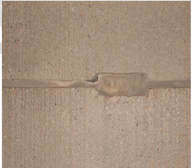
Photo 28 – Garage expansion area. Note sealant adhesion failure along filigree plank joint line.
