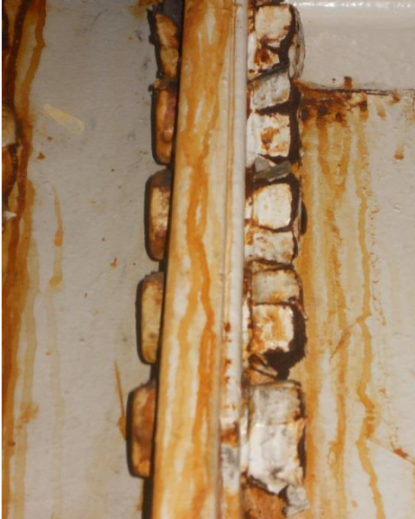
Photo 15 – Level 2 framing connection. Note corroded condition of high strength bolts and nuts.
