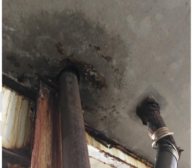
Photo 26 – Floor deterioration at drain line penetration. Note corroded condition of drain and line.
