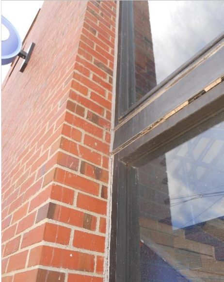
Photo 37 – Sealant deterioration at glazed curtain wall in stair tower #1
