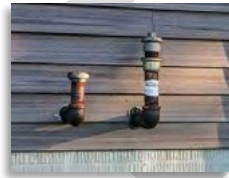
Oil tank pipes
