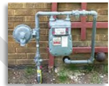
Natural gas piping
