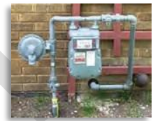
Natural gas piping
