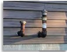
Oil tank pipes
