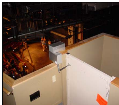
Accessible Lift Seacoast Repertory Theater
