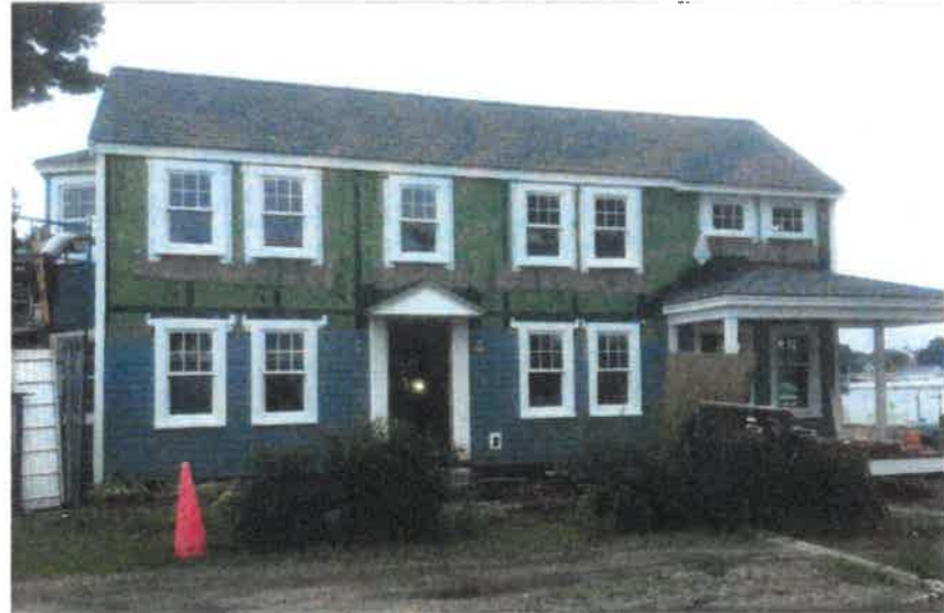
PHOTO OF INSTALLED 6/1
