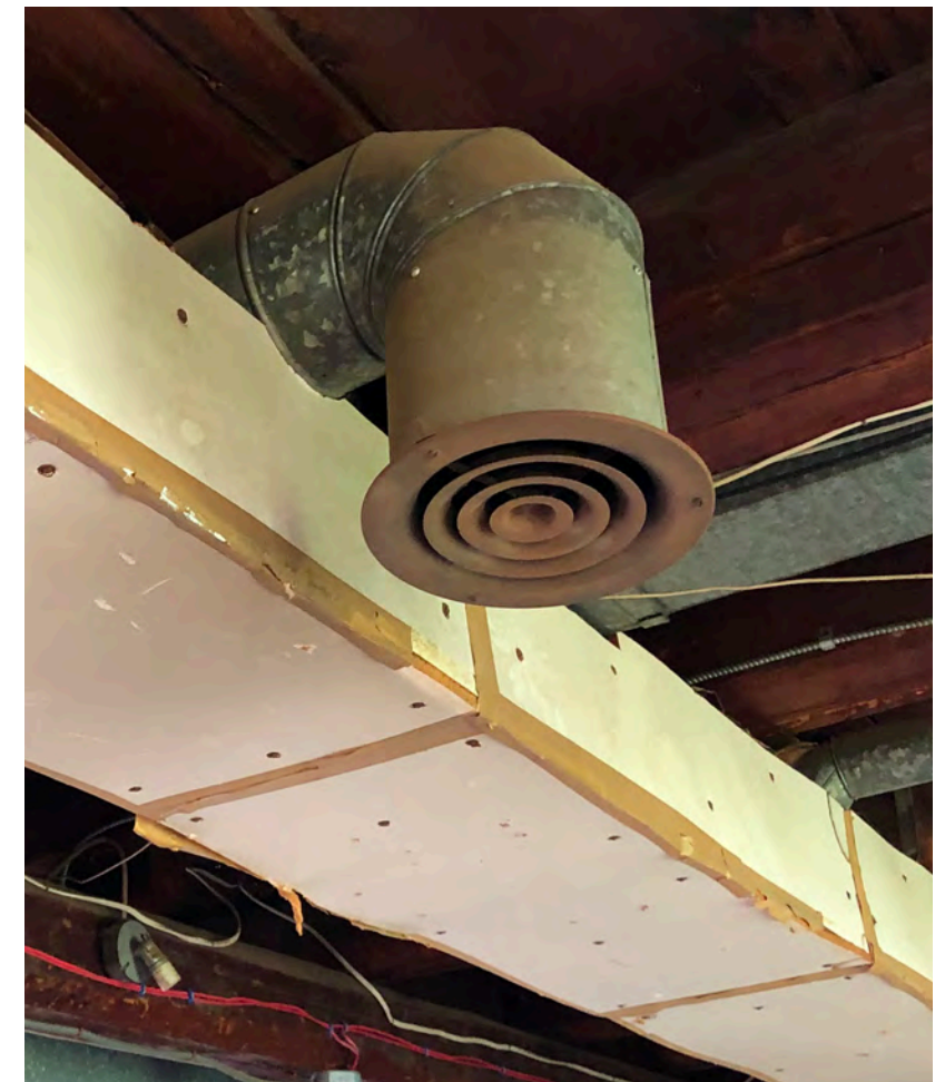
Shaw 1st Floor - HVAC DUCT
