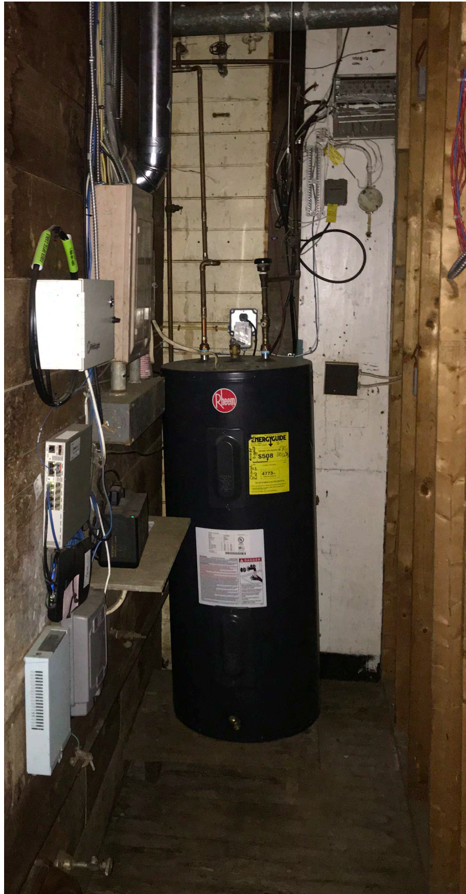
Shaw 1st Floor - Water Heater
