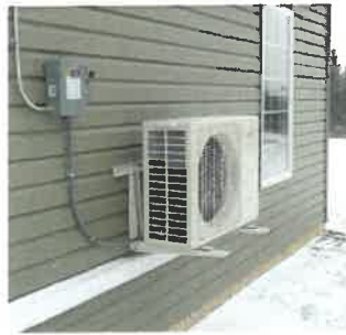
WALL MOUNTED HVAC EQUIPMENT- SIMILAR INSTALLATION
