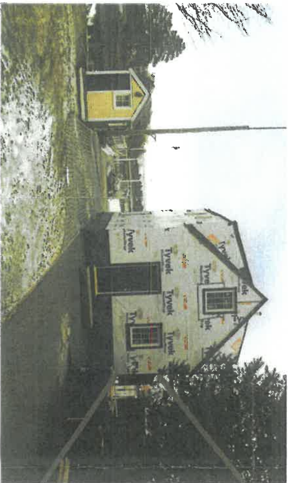
View Of Electrical Meter to be Relocated to Fence
