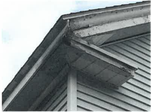
Aluminum Soffett/Peak Re-Wrap Project: Original aluminum covering to this area detached in storm exposing old wood. We would like to recover exposed wood with same material as existing to prevent further damage and infestation by bees and squirrels.
