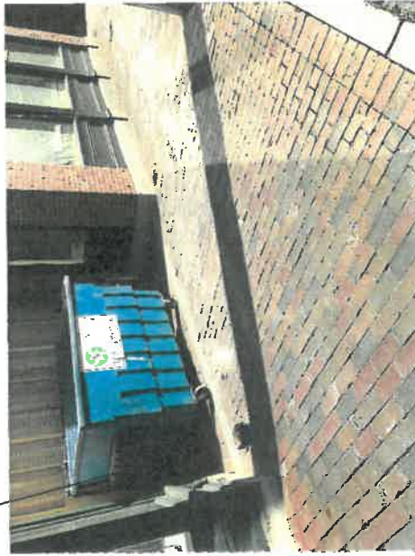
Brick pavers, to match adjacent sidewalk, with a granite band were installed per discussions with DPW.
