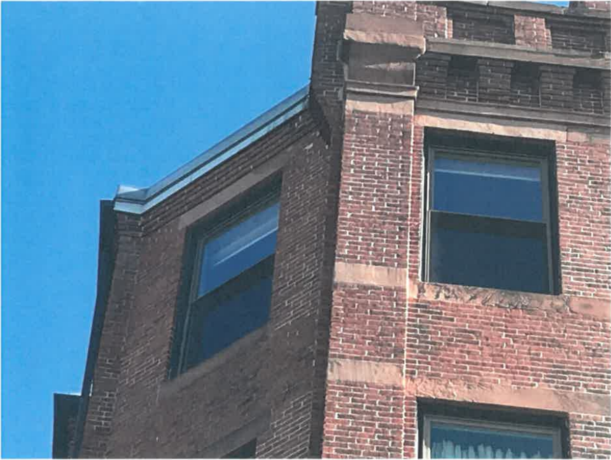
Next two photos show unit 501 with the Andersen window replacements - 5th floor top left unit.
