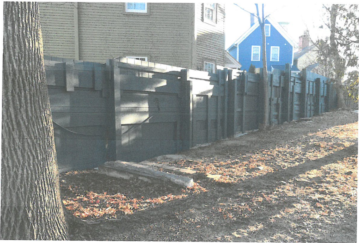
Existing back of fence, unfinished
