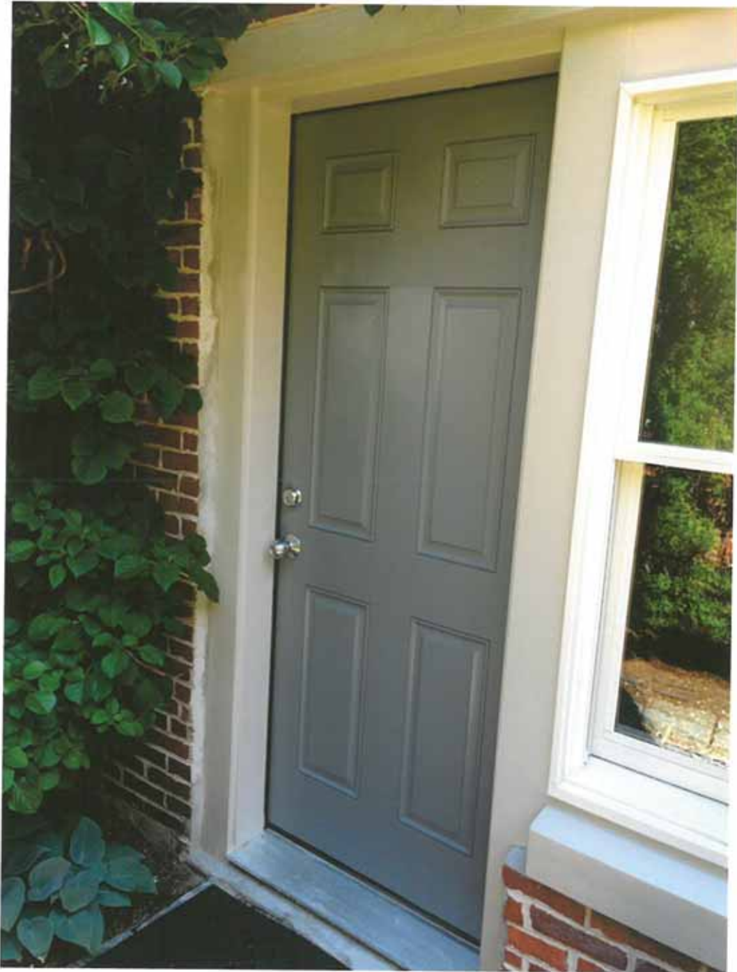
18 Sheafe Street — field painted door
