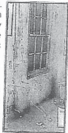
Thermal imaging shows that air leakage at the floor joint is much more significant than in the window.
